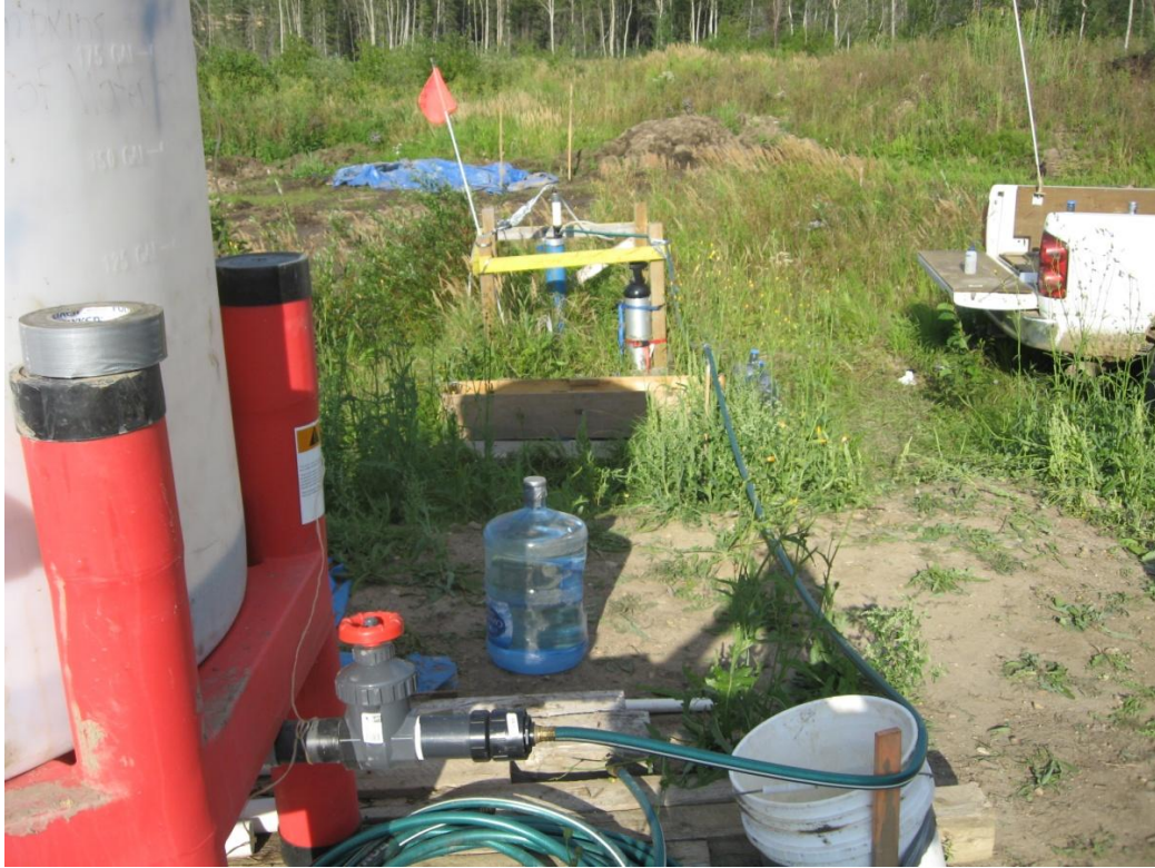
Figure 3-10: Injection System – Garden hose running from injection tank to STP-07-159-SS.
