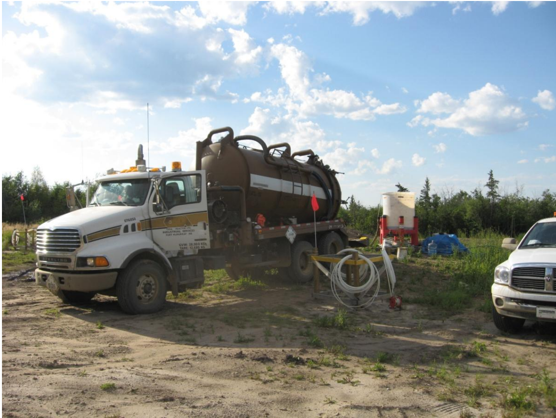
Figure 3-12: Transfer of PA water from vacuum truck to holding tank at the ISATF.
