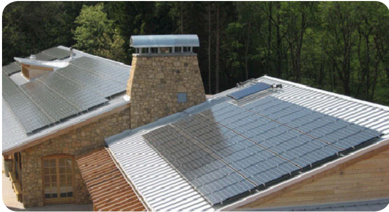
2.05 photovoltaic roof system
