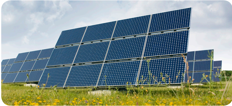
1.25 photovoltaics supplying renewable energy
