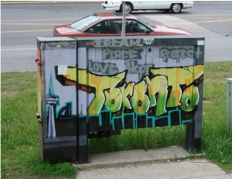
Fig 30. Graffiti by Style in Progress on Jane Street utility box.
