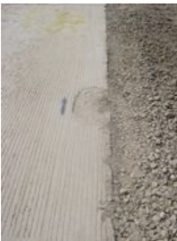
Figure 7.17 New Pothole in 0% Coarse RCA
