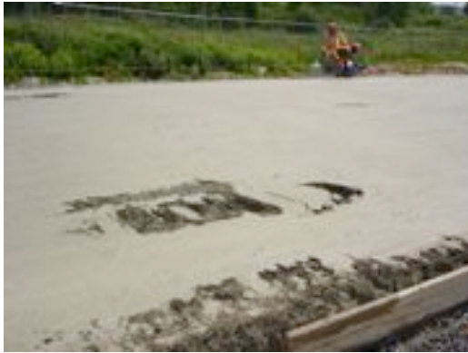
Figure 5.6 Condition of JPCP
