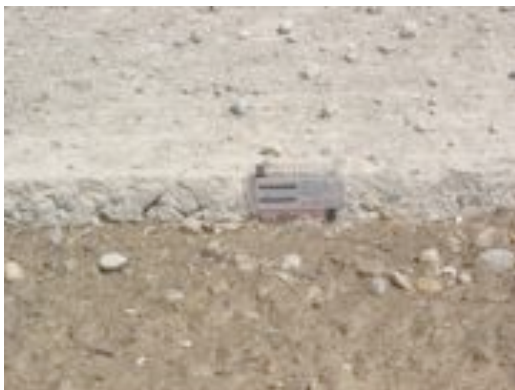
Figure 7.14 Pavement Edge Spalling and Shoulder Settlement
