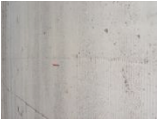
Figure 7.7 Transverse Depression from Slipform Paver
