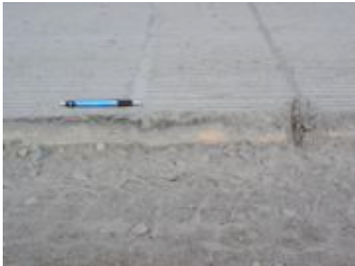
Figure 7.10 Pavement Edge Spalling and Shoulder Settlement
