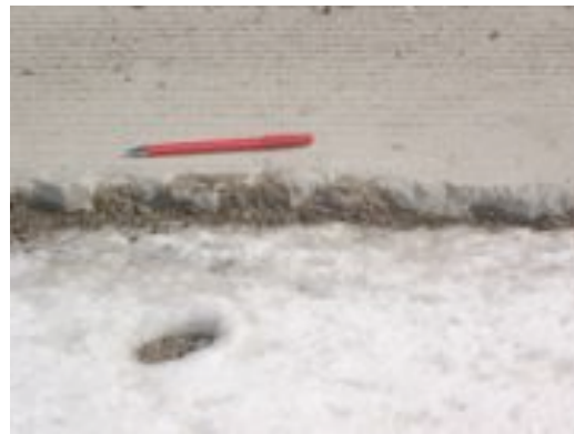
Edge and Shoulder Settlement
