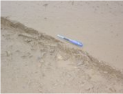
Figure 7.4 Pavement Edge Spalling and Shoulder Settlement
