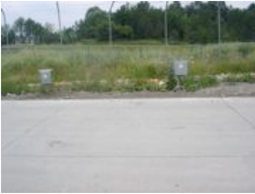
Figure 5.24 Location of Multiplexer and Datalogger Cabinets
