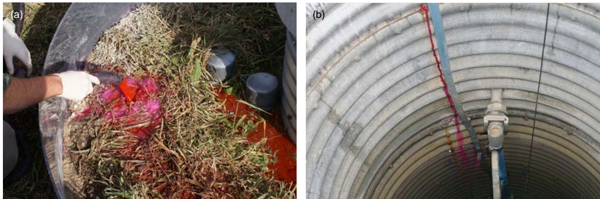
Figure 3.14. Photos of tracer solution at ETH3 (a) being placed on thick grass cover, and (b) leaking through the riveted seam in corrugated galvanized casing.
