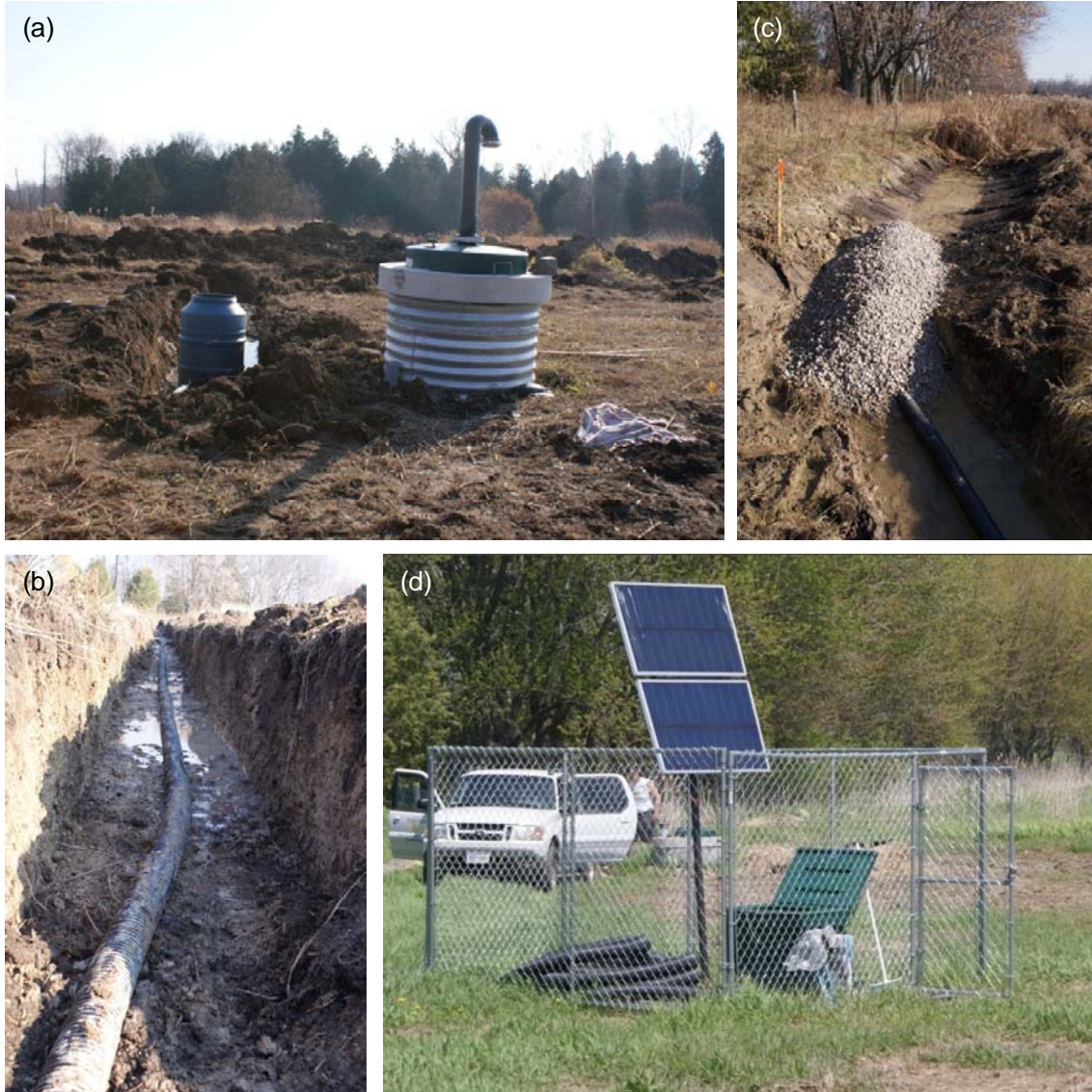
Figure 2.8. Drainage system photos showing (a) sample collection facility for ETH3, (b) drainage line from sample collection facility, (c) drainage line and stone cover at drainage ditch, and (d) solar panel and electrical enclosure.
