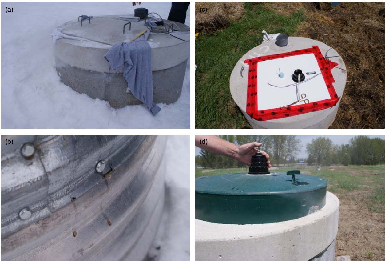
Figure 3.8. Photos of smoke tracer tests showing (a) rags used to seal CTH1 during test #1, (b) dark coloured water leaking from seams of ETH3 casing during test #1, (c) apparatus properly sealing CTH1 during test #2, and (d) smoke escaping from Poly – Lok lid of ETH1 during test #2 caused by damage during test #1.
