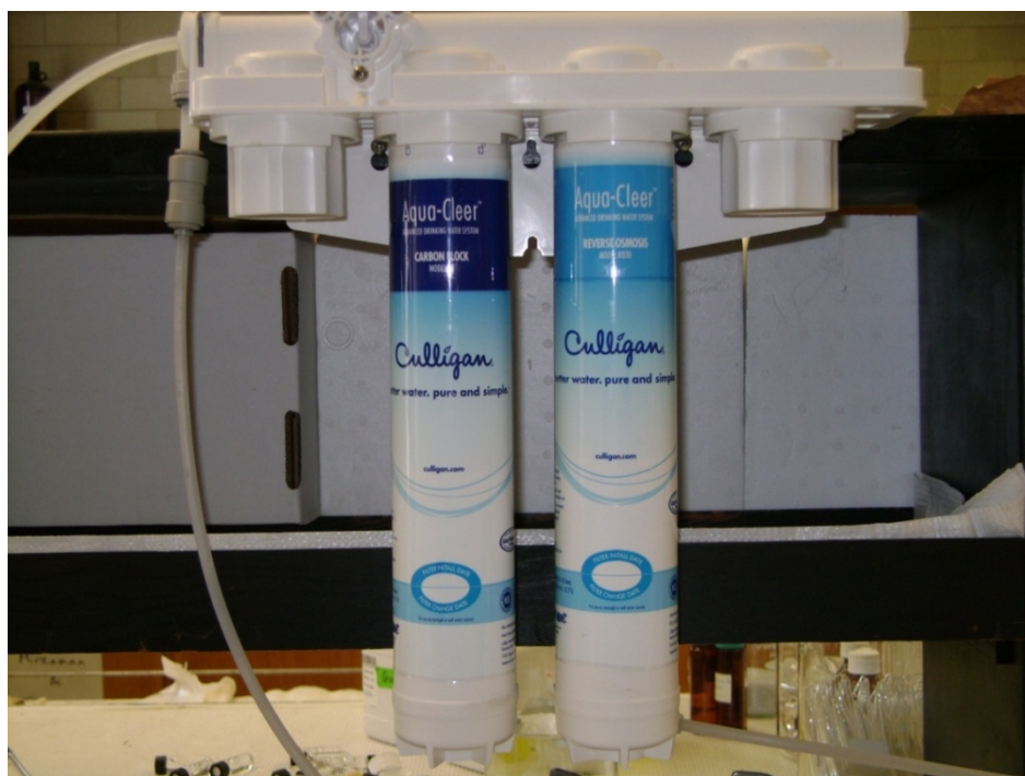
Figure 3-5: RO membrane preceded by only carbon block.
