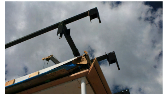
fig 2.5.7 corner showing end brackets on roof racking frames and purlins
