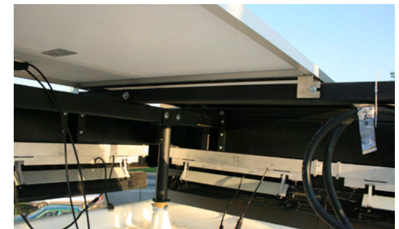
fig 2.14.7 close up of solar panel bracket as installed
