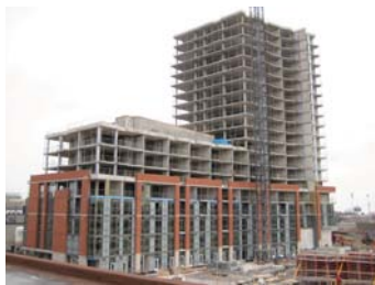
Fig. 10.12 Construction of the first of two West Side Lofts buildings is well underway.
