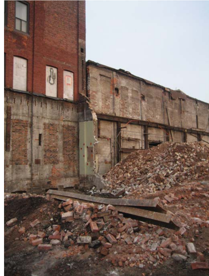
Fig. L.6 Rubble in the place of IMAR steel's old unit.
