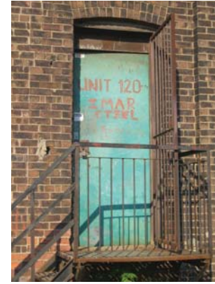
Fig. J.3 IMAR Steel was evicted from Abell's west wing in November 2007.
