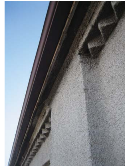
Fig. 7.7 Above, Stucco applied to some exterior walls of 48 Abell caused possible moisture damage to the brick according to report.
