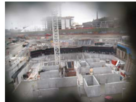
Fig. 10.15 New foundations poured at 48 Abell's former west wing. View from a hole in the window of building stairwell.
