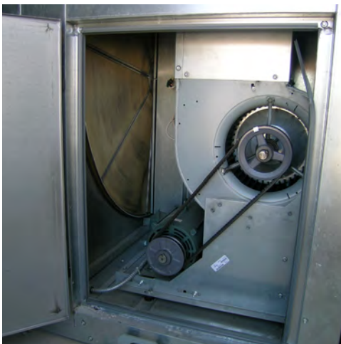
Figure 4.5.31 Heat-recovery using an enthalpy wheel at Artists for Humanity
