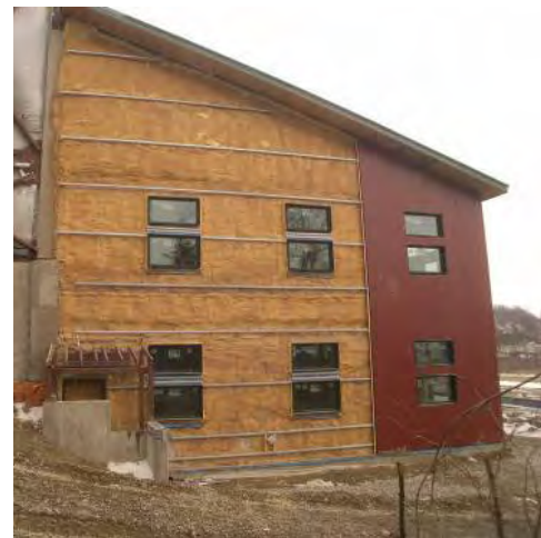
Figure 4.5.21 West wall at Wind NRG, Phase 2 Openings are similar to Phase 1 which the WWR, west, is 16.4% (image Maclay Architects 2008)
