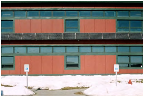
a (top): brick at T.L. Wells b (middle): wood siding at Holyrood RCMP c (bottom): metal siding at Wind NRG
