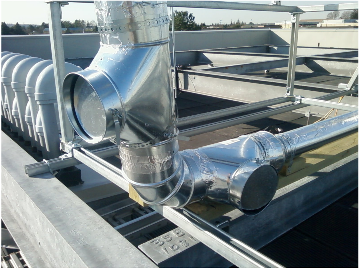
FIGURE 4.11 DUCTS FOR TEMPERATURE CONTROL
