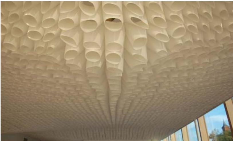
Figure 2.24: Detail of the suspended fabric ceiling panels
