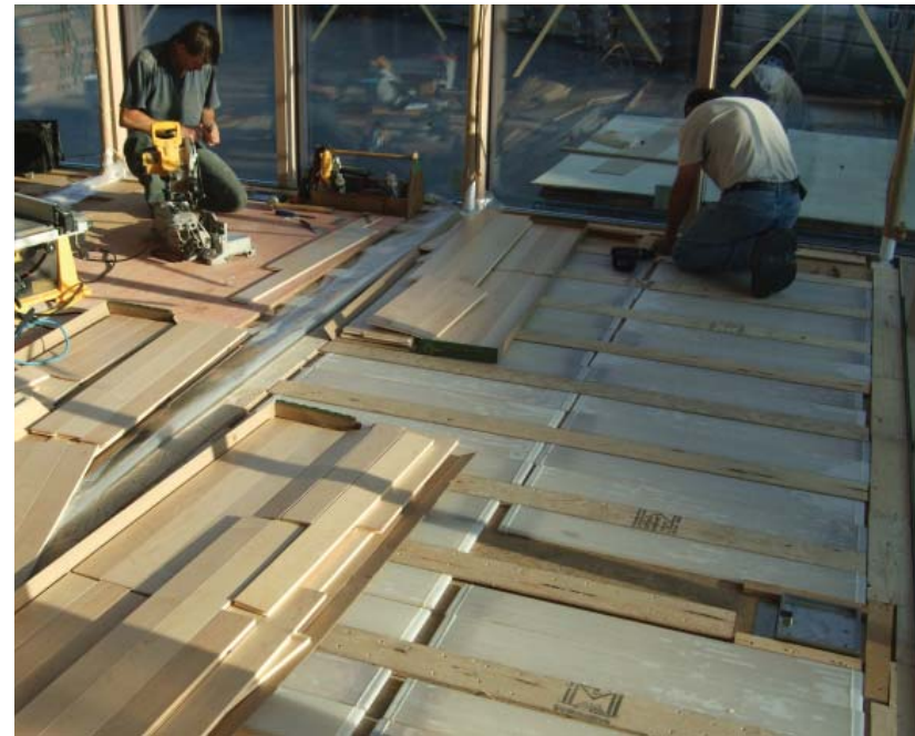
Figure 2.22: Salt Hydrate Phase Change Materials (Delta-Cool 24) are laid over the sub-floor, alternating with plywood battons supporting the engineered maple hardwood floor.
