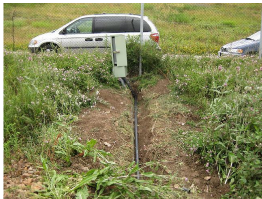
Figure 48 Conduit with Cables Running to Data Logger
