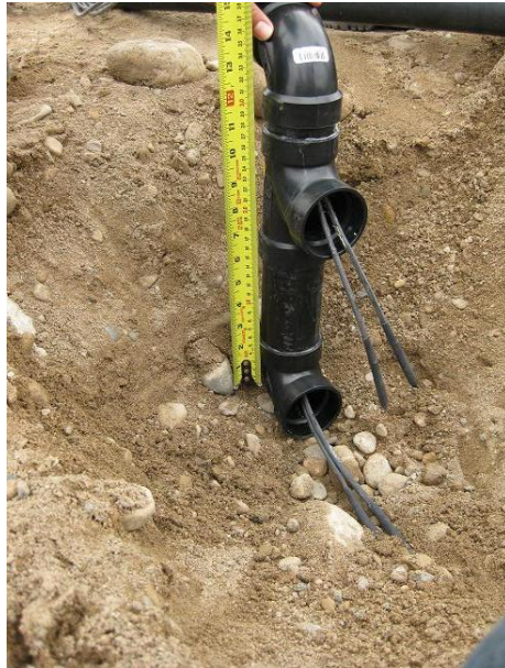
Figure 34 Temperature Probes in Sensor Tree
