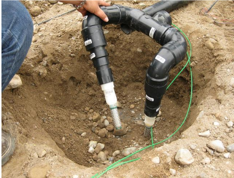
Figure 30 Moisture Sensors in Sensor Tree in Second Phase
