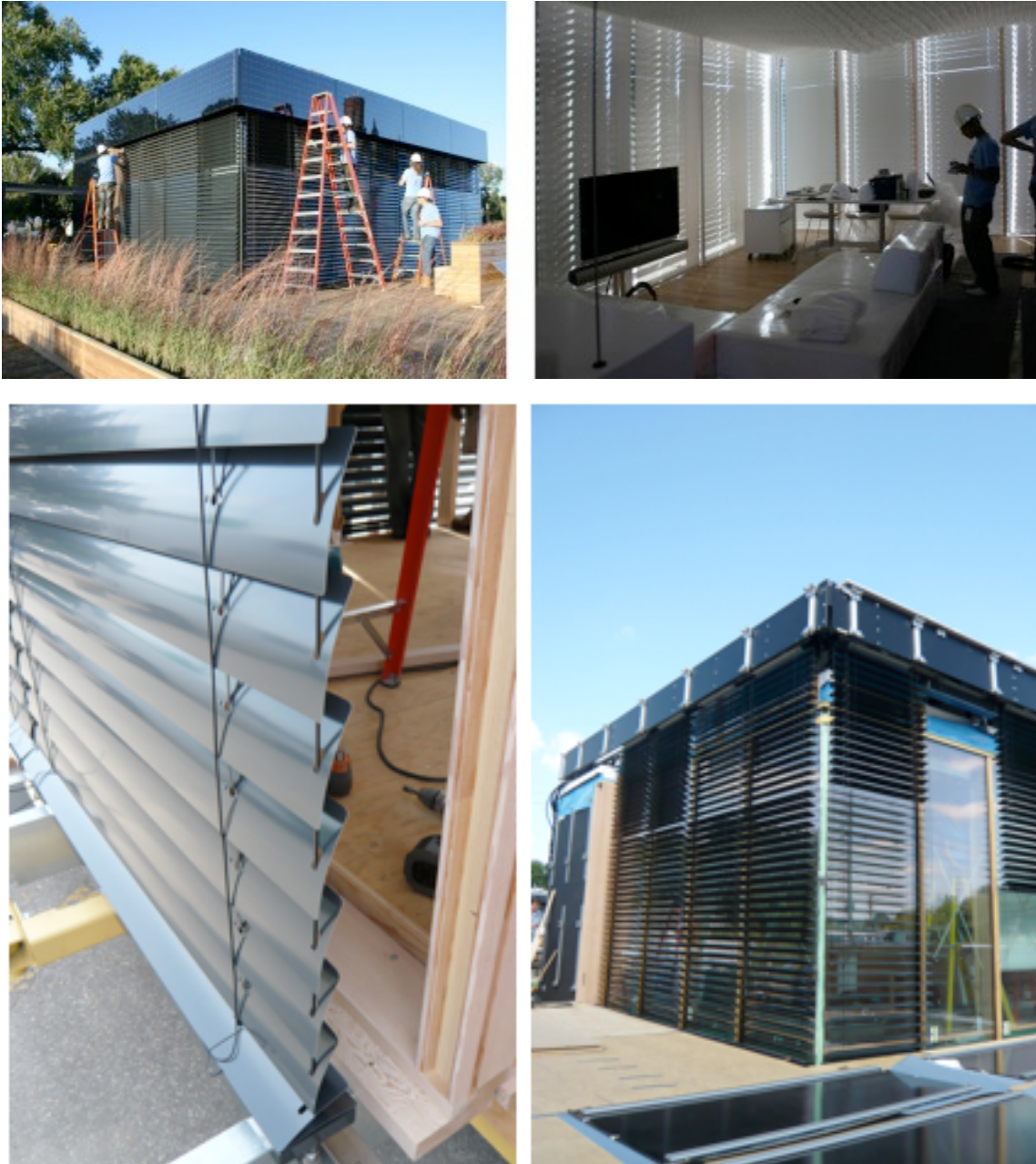
Figure 2.2.5 Exterior venetian blinds and interior roller blinds of North House
