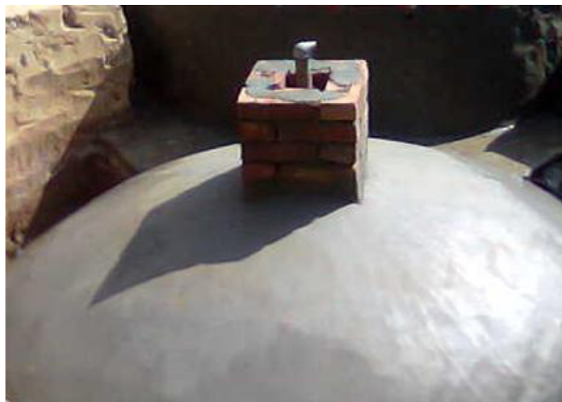
7.10. Photo of the top of a bio gas plant
