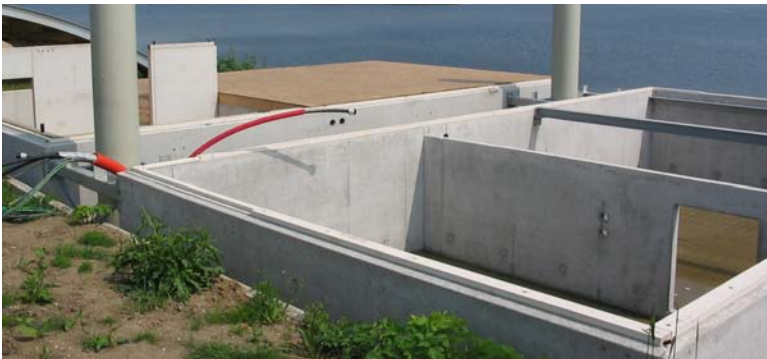
5.6. Concrete foundations, poles and flexible plumbing connections
