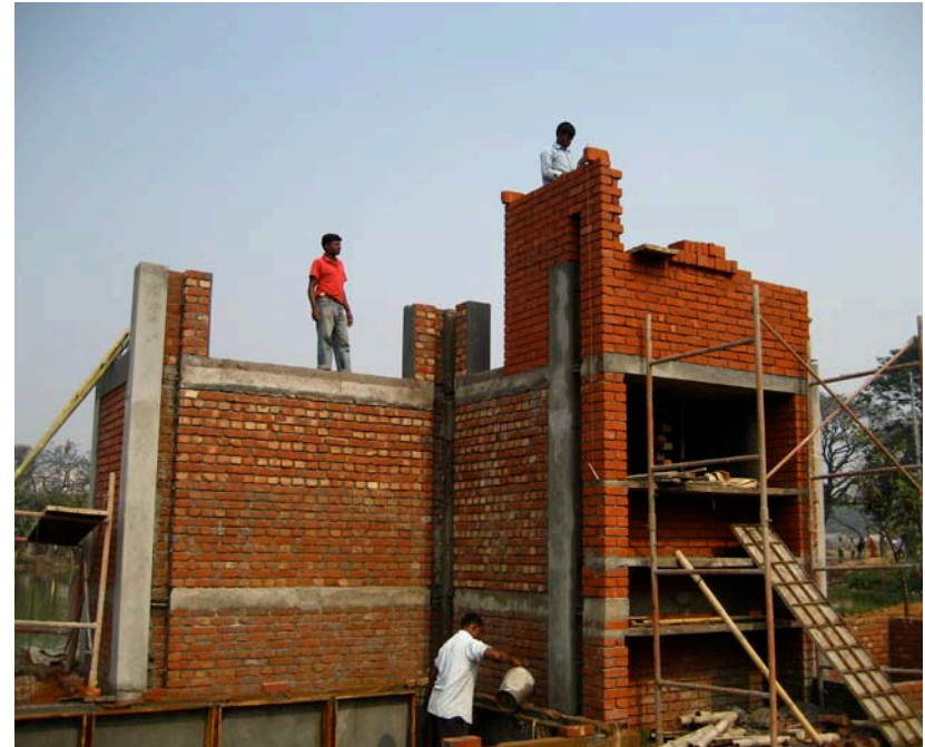
8.75. Grooves left in wall of the service spine to place vertical guidance tracks
