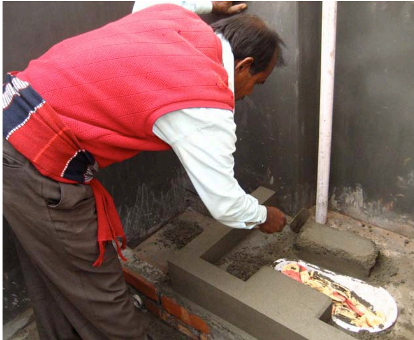
8.96. Custom latrine made to divert urine
