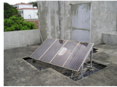
c. Photovoltaic System
