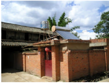
a. Solar Water Heater
