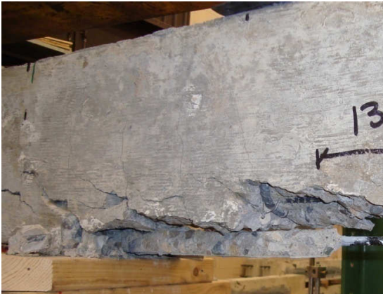
d-Region 3 with concrete chunks separated from the beam
