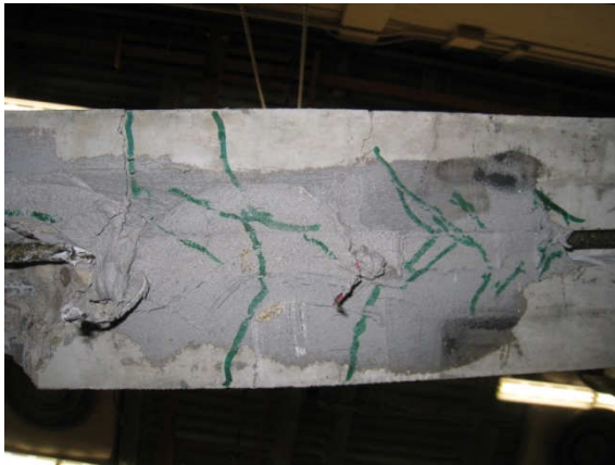
a-Cracks fanning from the CFRP rod
