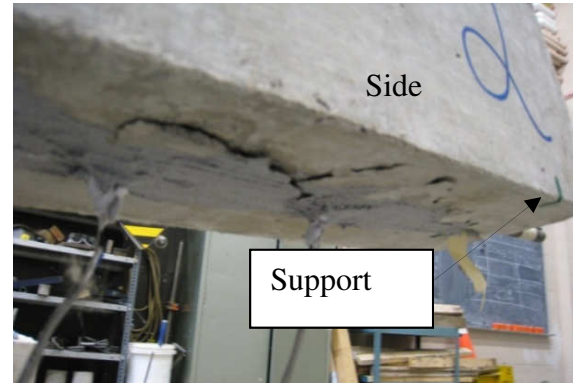
c- Longitudinal cracks in the epoxy and the
