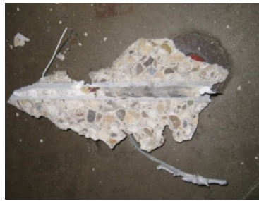
c-Epoxy with concrete separated from the bottom of the beam
