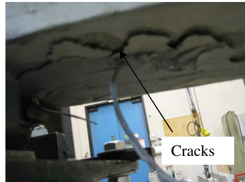
b-Cracks in concrete surrounding the epoxy
