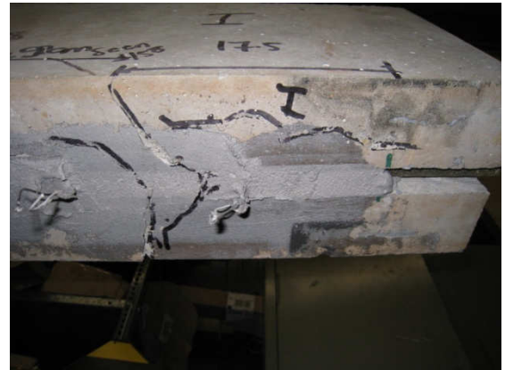
b-Cracks parallel to the CFRP rod
