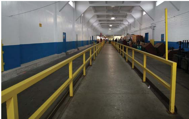
4.20 Existing interior road conditions within the main Terminal building accommodate small motorized carts and forklifts on the left and right sides. A central path for pedestrians is marked with guardrails.
