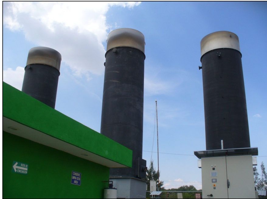
Figure 4.11: BIOGAS flares that cleanly burn methane. Only the flare on the right was in use when this picture was taken. The flares, which were designed in the UK, convert methane to carbon dioxide at an efficiency of 99.9999%.
