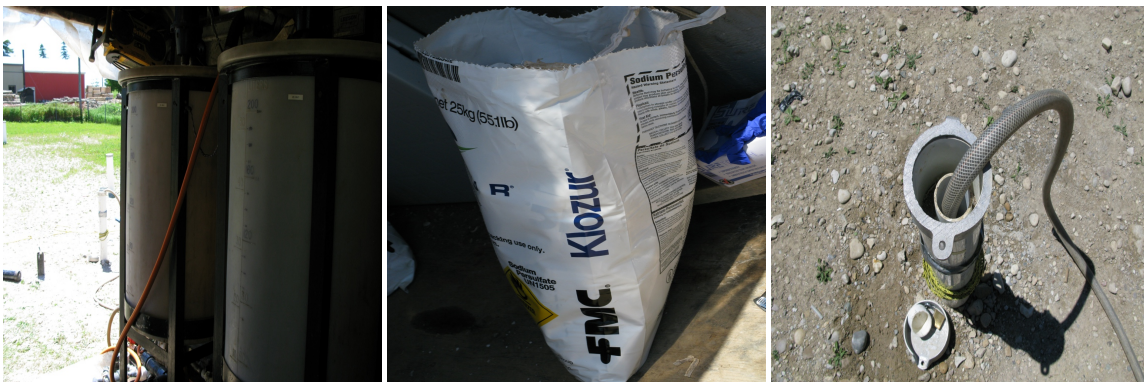
Figure 12. 100L mixing tanks, FMC sodium persulphate, 2-inch PVC injection well
