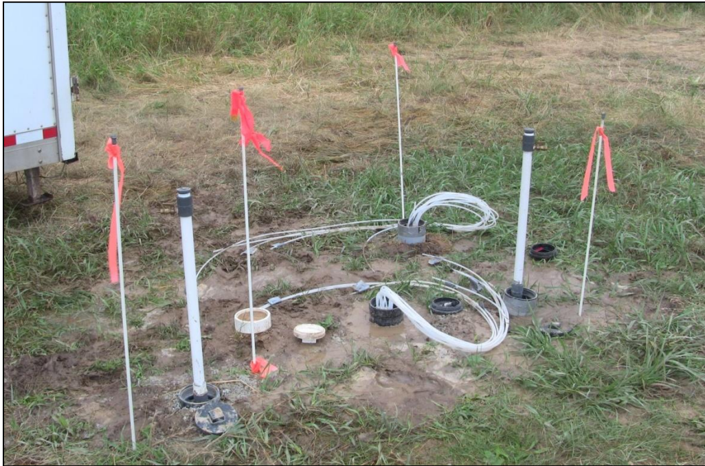
North Campus Injection site wells (looking north)
