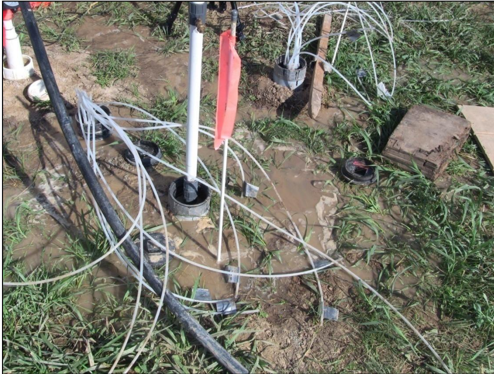
Water pooling at ground surface during injection
