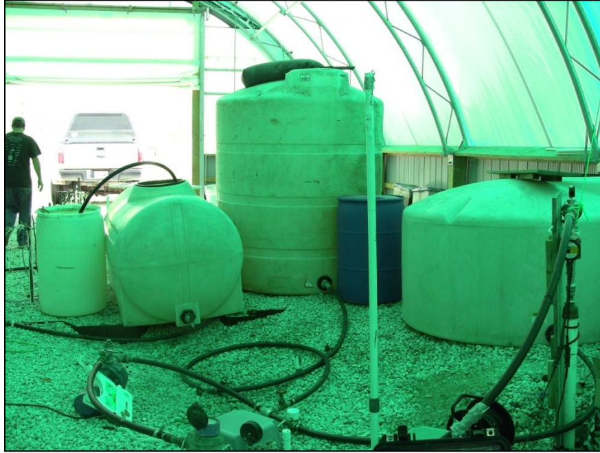
Holding tanks used to store tracer solution at surface (total 7500 L capacity)
