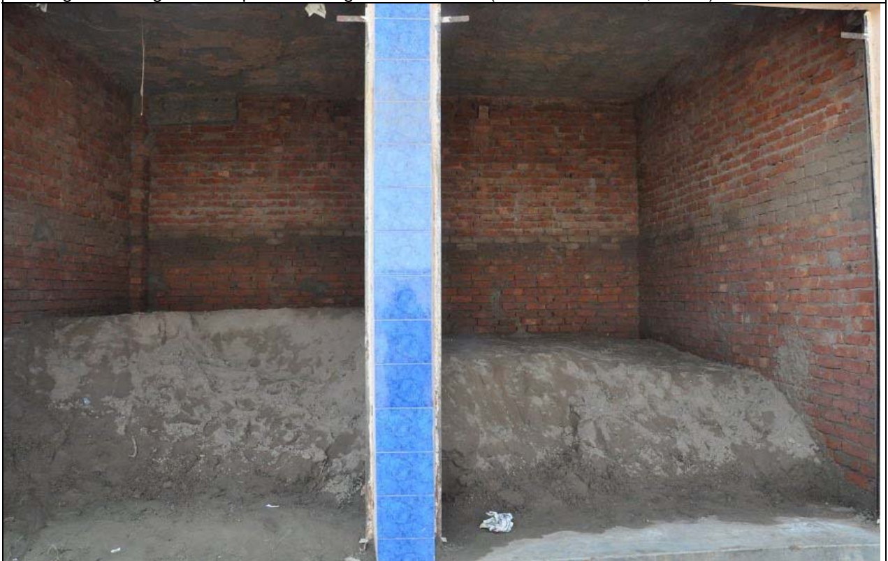
Silt deposited in the shops after the floodwater receded (Source: MinaAllah, 2010b).
