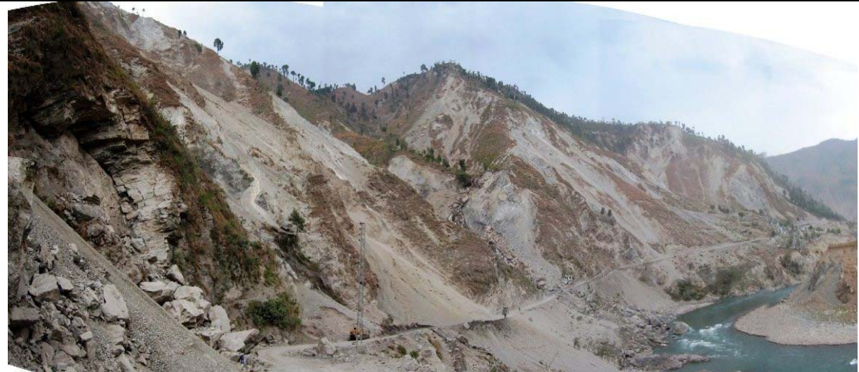
Extensive land sliding along the road in Muzaffarabad (Source: Durrani et al. , 2005).
