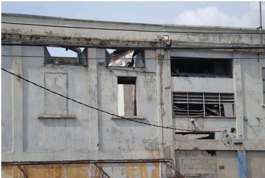
Fig. 1.14 LEFT - View of the decaying facade of a vacant building in Downtown, Kingston.
