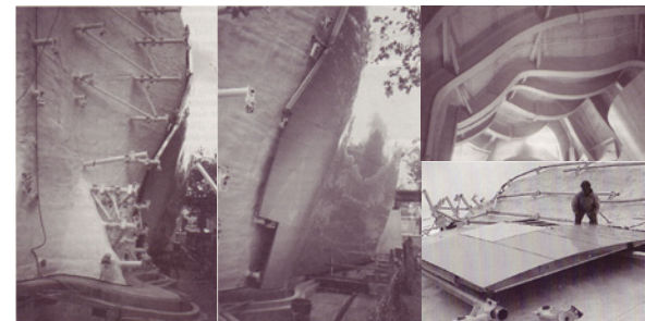
Figure 2.1-10 The complex curvilinear metal panels that clad Gehry Partners' Experience Music Project were installed with the assistance of GPS satellite guidance.
