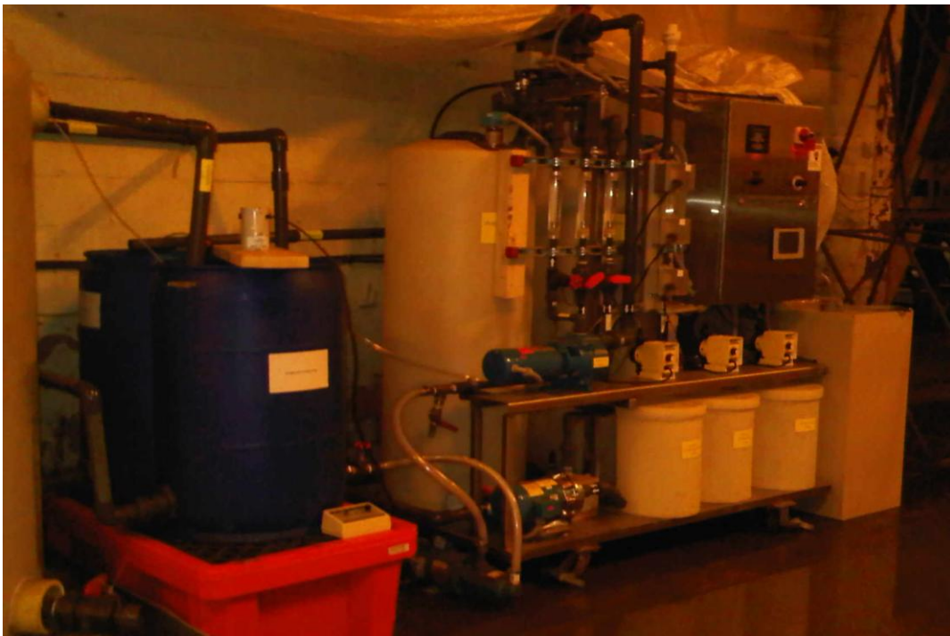
Figure 3-7 A picture of the pilot plant as installed and operated at the factory
