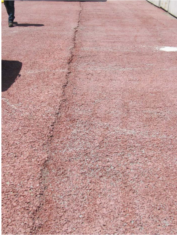
Figure 5-13: Construction Joint A/B at Site 4 June 2010 (20 Months)
