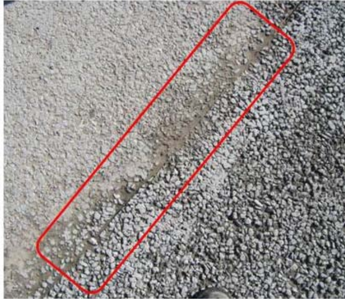
Figure 5-10: Saw Cut Joint Site 5 June 2011 (32 Months)
