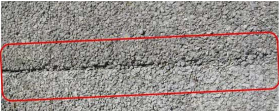
Figure 5-5: Formed Joint August 2009 Site 1 (26 Months)
