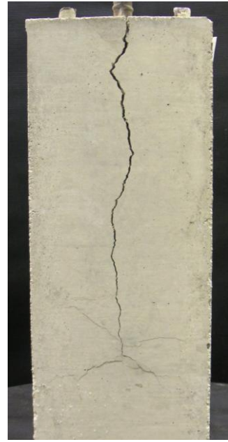
b) Post-failure cracking
