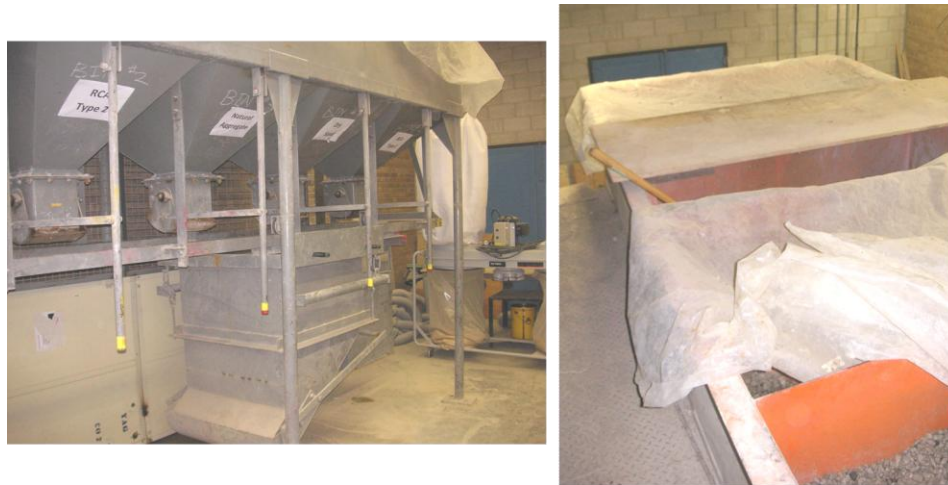
Figure 5.2 Aggregate hopper systems and pre-wetting of coarse aggregates in hoppers as per batching methods B and C
