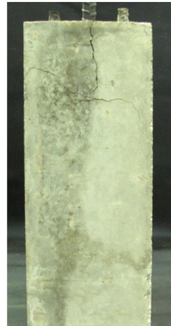
b) Post-failure cracking
