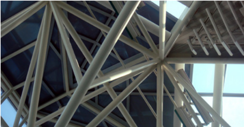
[3.1.22] A view of the bulky space frame structure of the roof above the security checkpoint.
