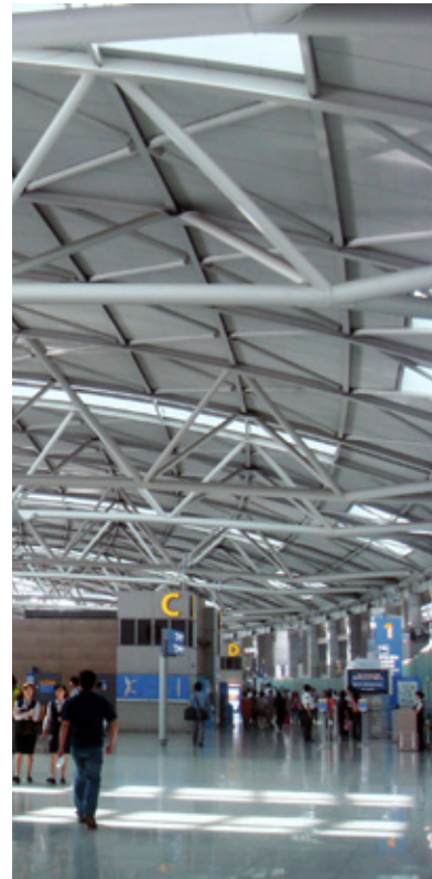
[3.1.5] The trusses of the check-in hall seem excessive in size and distract from the elegant sectional shape.
