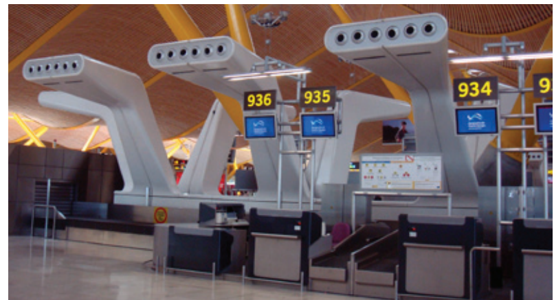
[3.41] The HVAC system has been integrated into the check-in stands to promote air circulation at the passenger level.
