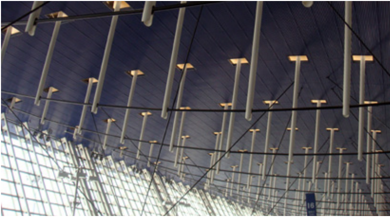
[3.1.12] The blue roof structure of Pudong's T1 works both in tension and compression.
