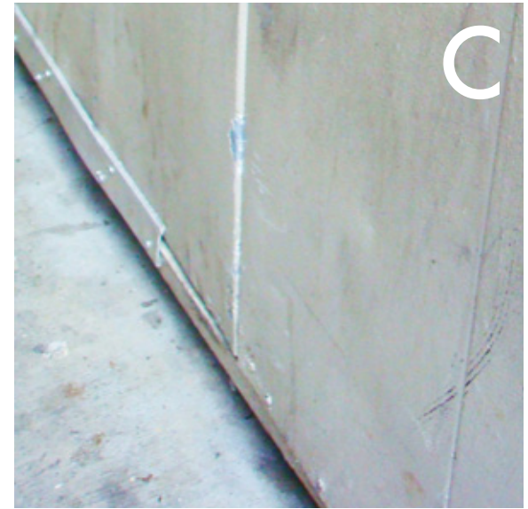
[2.17] Damaged stucco exterior at John F. Kennedy Airport Terminal 2.
