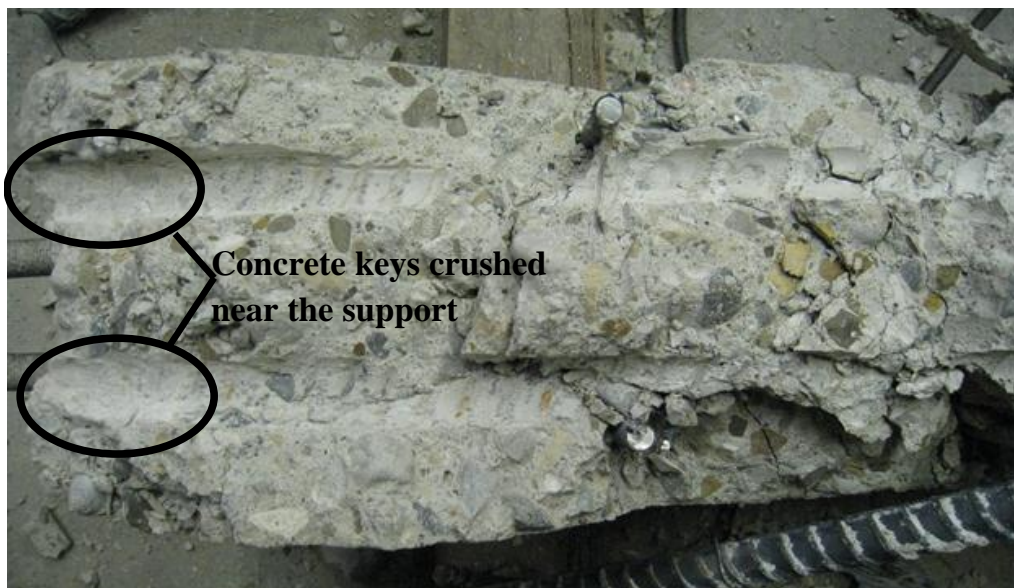
Figure 4.38 Beam F-A-66-0 after failure and reinforcing bars removed. The beam is turned upside-down.
