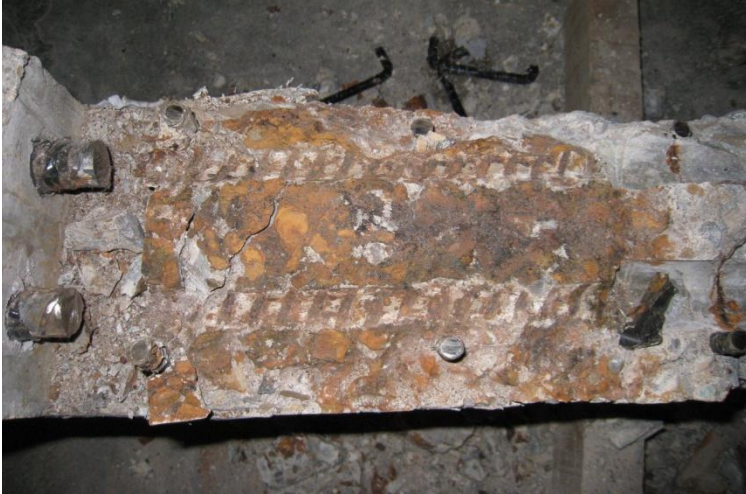
Figure 5.20 Beam M-200-U-m after failure and removing the reinforcing bars to examine the concrete keys. The beam was turned upside down.
