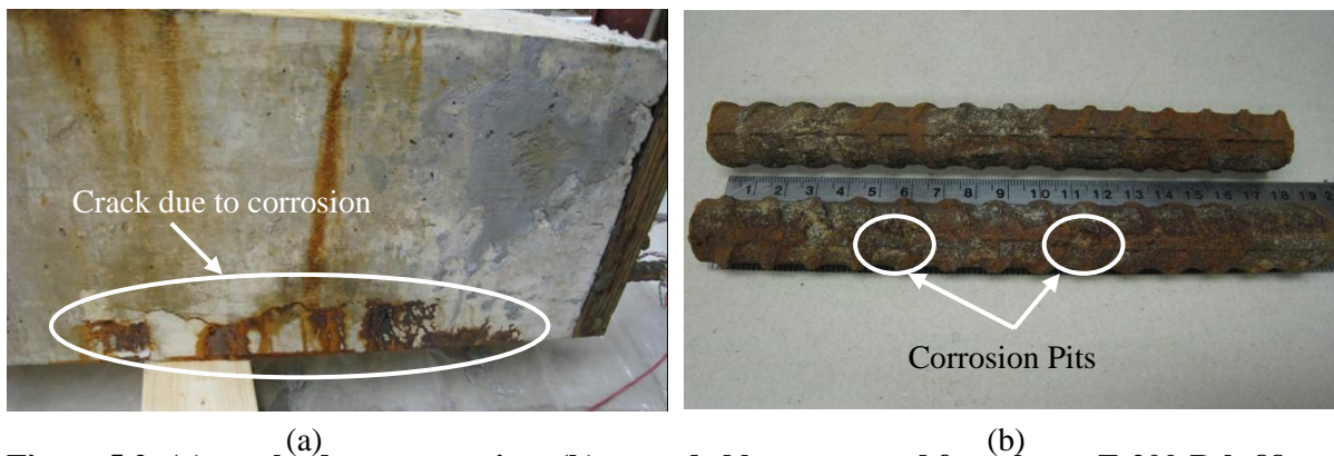
Figure 5.2: (a) cracks due to corrosion; (b) corroded bar extracted from beam F-200-R-h-88.
