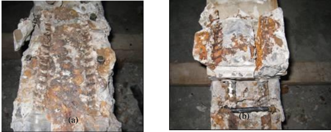
Figure 5.45: (a) upper concrete above bar and (b) lower concrete below the bar in beam F-200-U-m-43.
