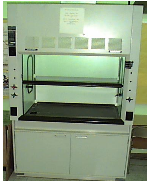
Figure B. 1 Chemical fume hood
