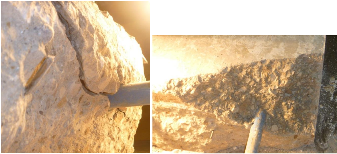
Figure 6-13 – Pilot slab Cracking at dowel
