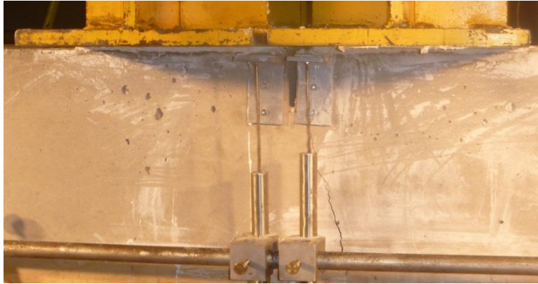
Figure 6-9 – Pilot Test Slab Crack Formation at 60 kN
