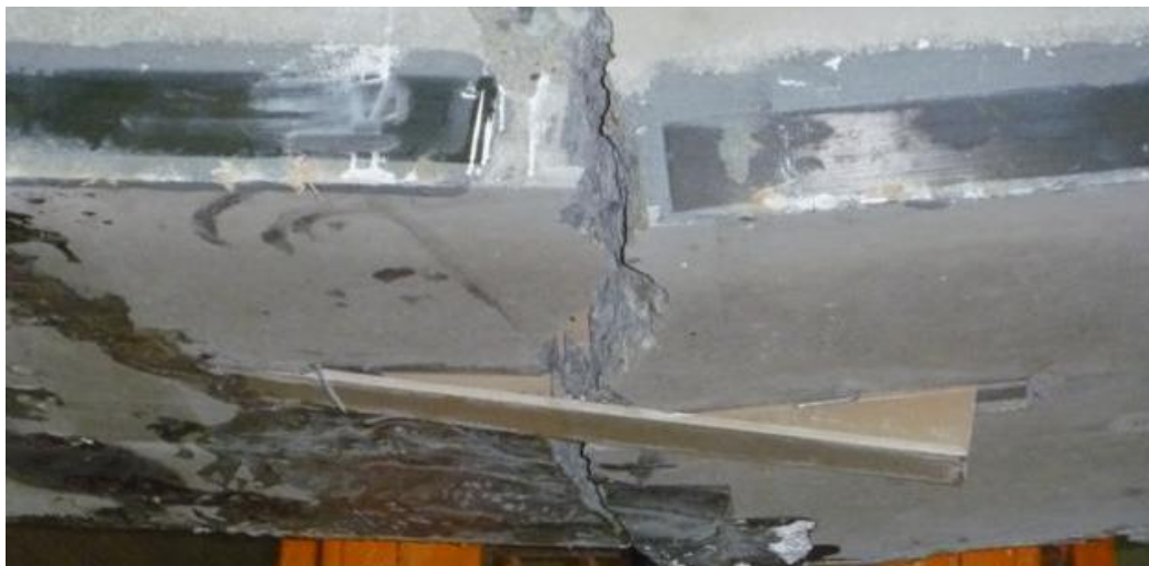
Figure 6-28 –GFRP I-Beam Specimen: GFRP I-Beam Penetration through Slab at Failure
