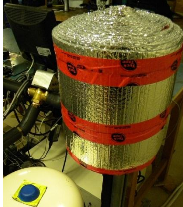
Figure 3.15 Hot water buffering tank in heat pump inlet branch
