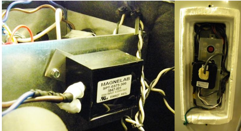
Figure 3.19 Heat pump voltage transformer (left) and DHW tank current sensor (right)
