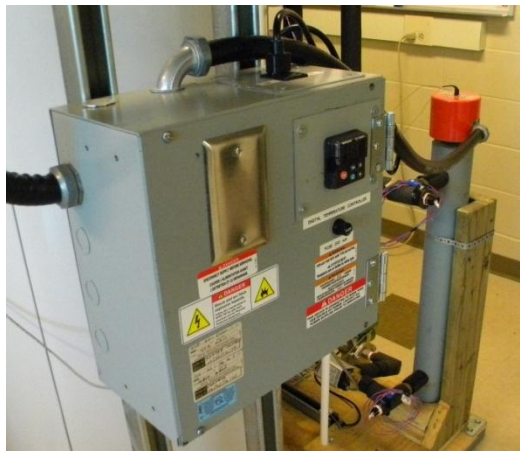
Figure 3.9 Circulation heater and power switching electronics box
