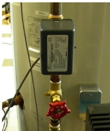
Figure 3.8 Floating point electronic valve with gate valve for simulated hot water draw
