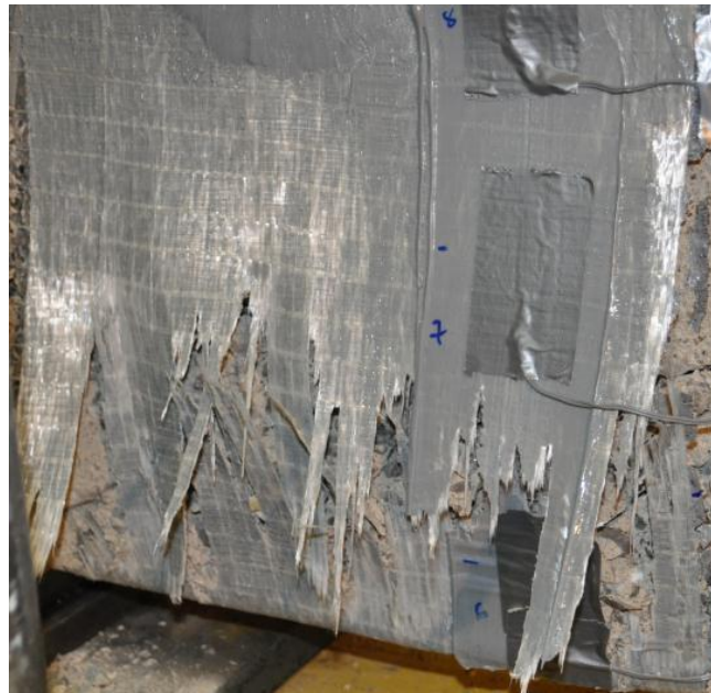
Figure 2-10: Ruptured GFRP u-wrapped sheet
