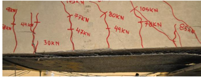
Figure 2-16: Plate end debonding
