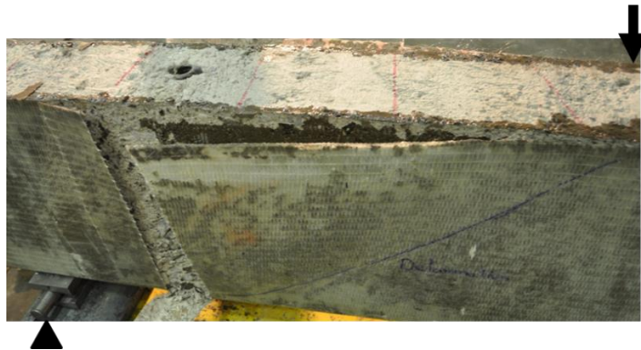
Figure 5-10: FRP debonding failure of beam 100G-1100-NA
