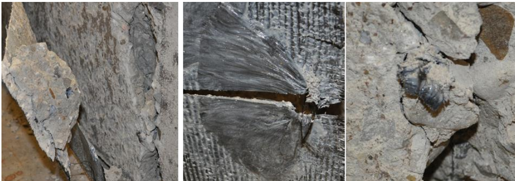
Figure 6-16: Concrete cone anchor failure and anchor rupture
