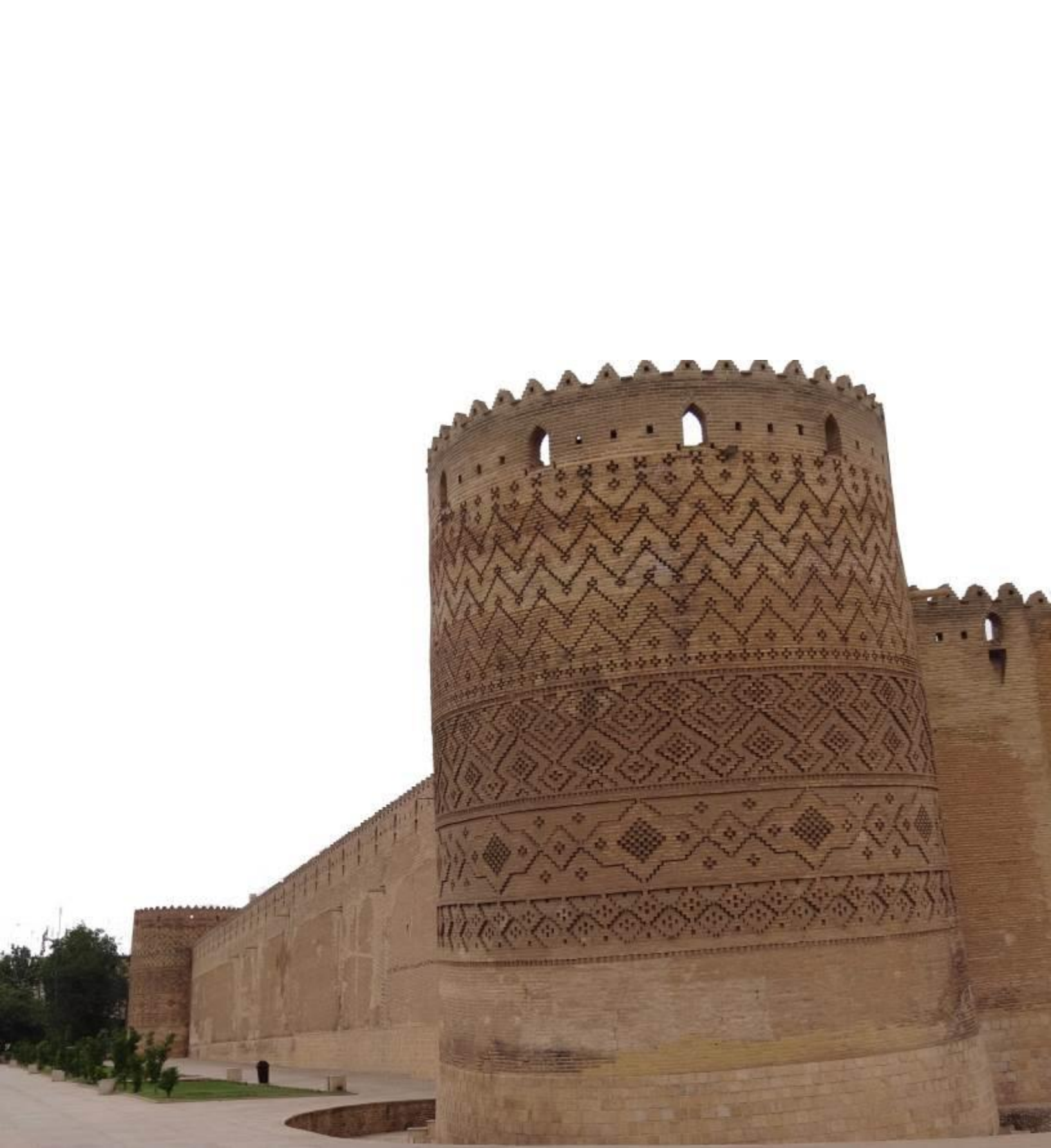
Fig 1.62 - Leaning Tower and Wall – Karim Khan Citadel, 18th century Shiraz, Western Iran
