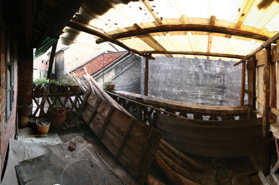
The balcony, with sheet plastic roofing to cover the lightwell to the kitchen below.
