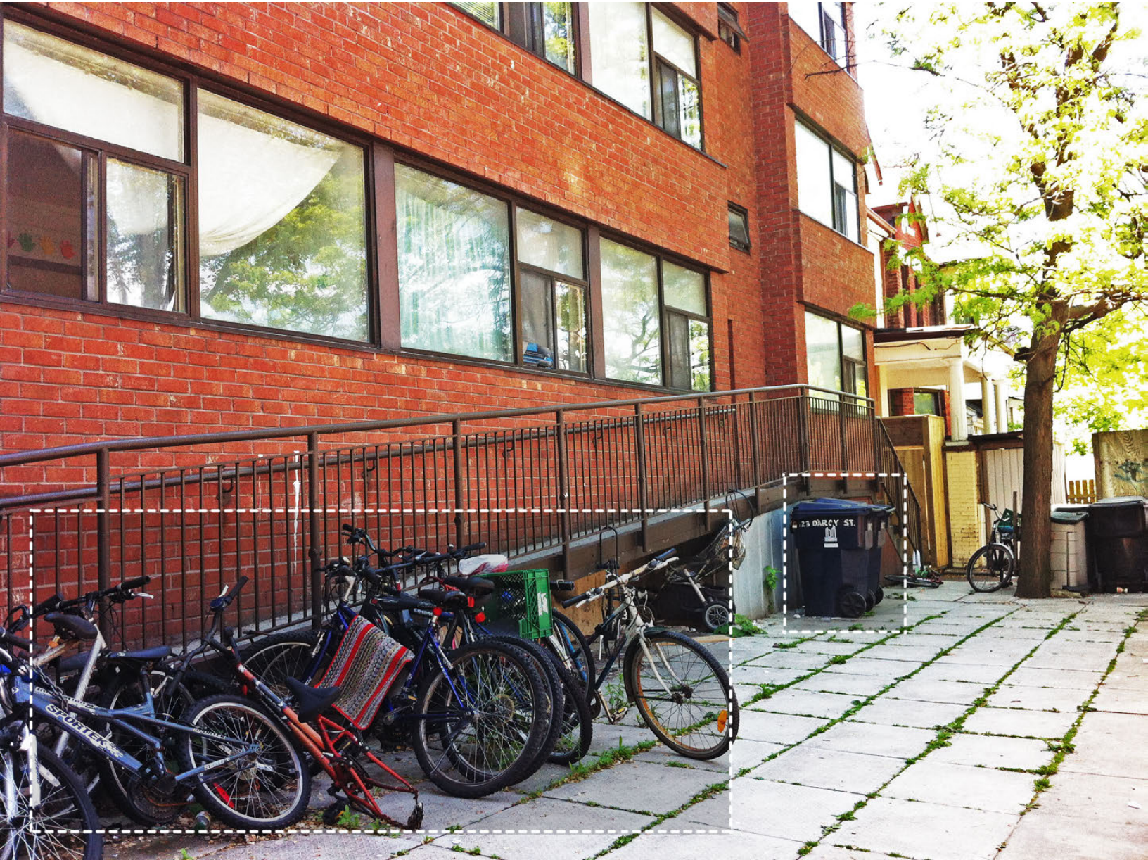
Fig 2.09: View to the apartment entrance from D'Arcy Street. Bicycles are piled in front the ramp since the railings are perfect for locking the bikes to. No proper space for garbage bins.
