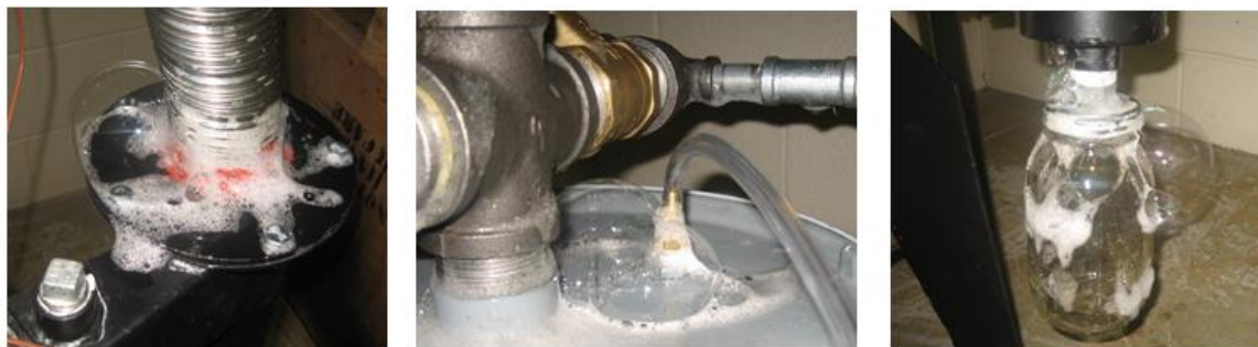
Figure 19: Identifying the leaks using the pressure test and soapy water
