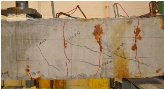
b) Low corrosion level beam D12-7.5%-UR
