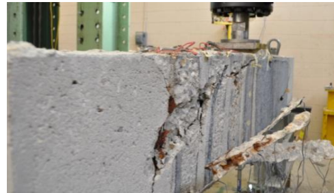
Close up on delamination of concrete cover
