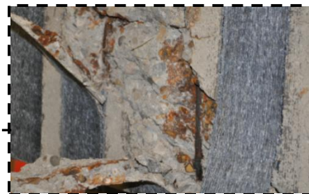
Close up on delamination of concrete cover
