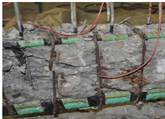
Figure 2.12 Stirrups after removing concrete cover
