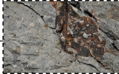
Close up on diagonal crack with stirrups rupture
