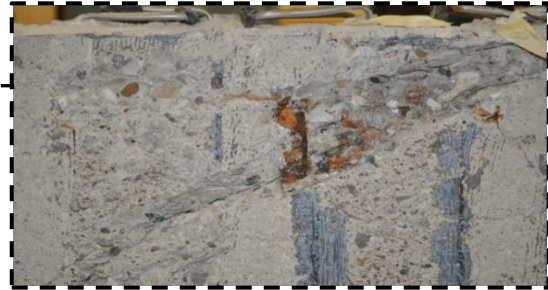
Close up on diagonal crack causing FRP debonding
