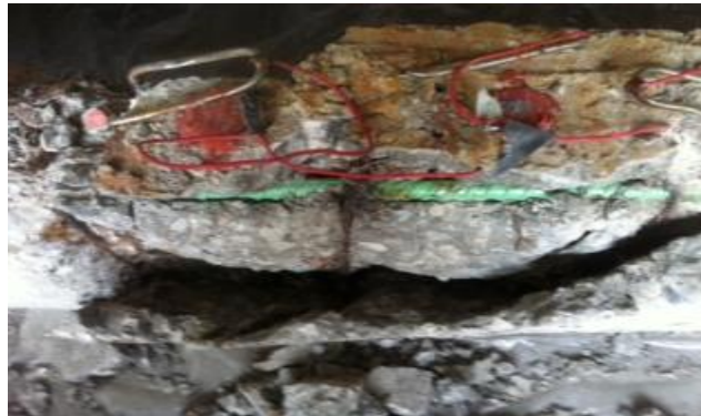
Figure 4.9 Concrete cover delamination as one layer due to corrosion damage on the stirrups (top view of corroded beam)
