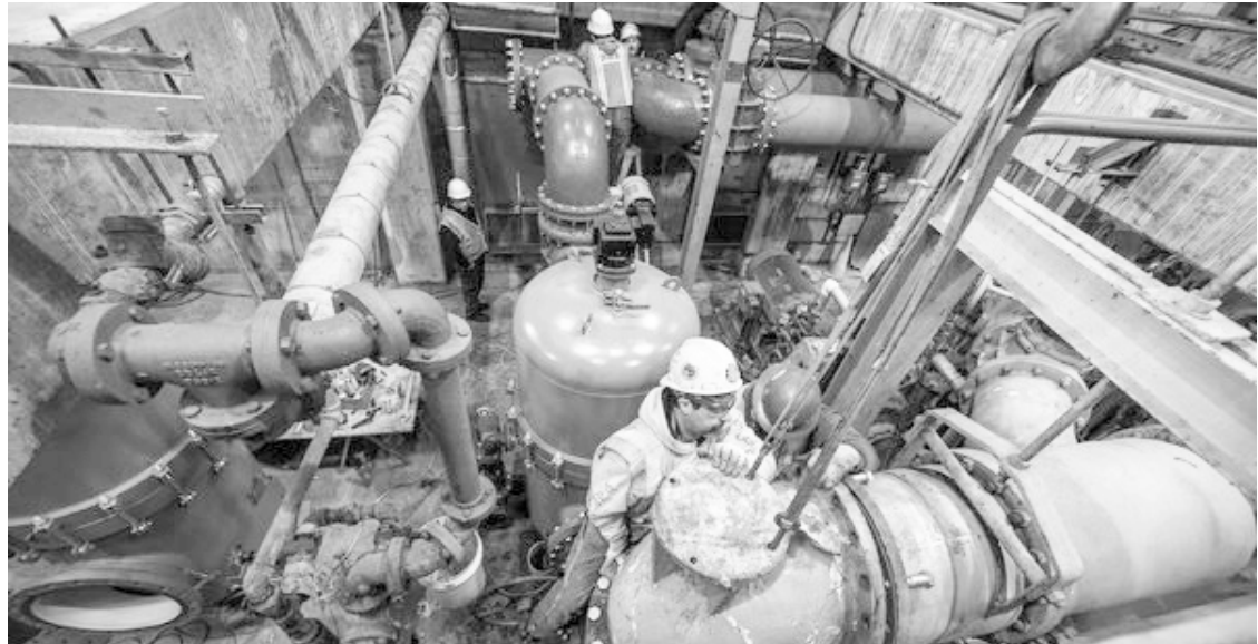
Fig. 3.1 Workers replacing damaged pumps at the Bay Park wastewater treatment facility in East Rockaway, New York.
