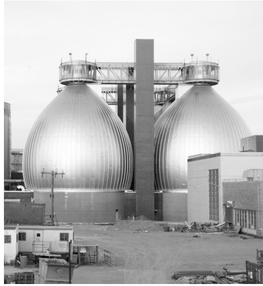
Fig. 3.9 The iconic anaerobic digestors of the New York City's Newton Creek Wastewater Treatment Facility.
