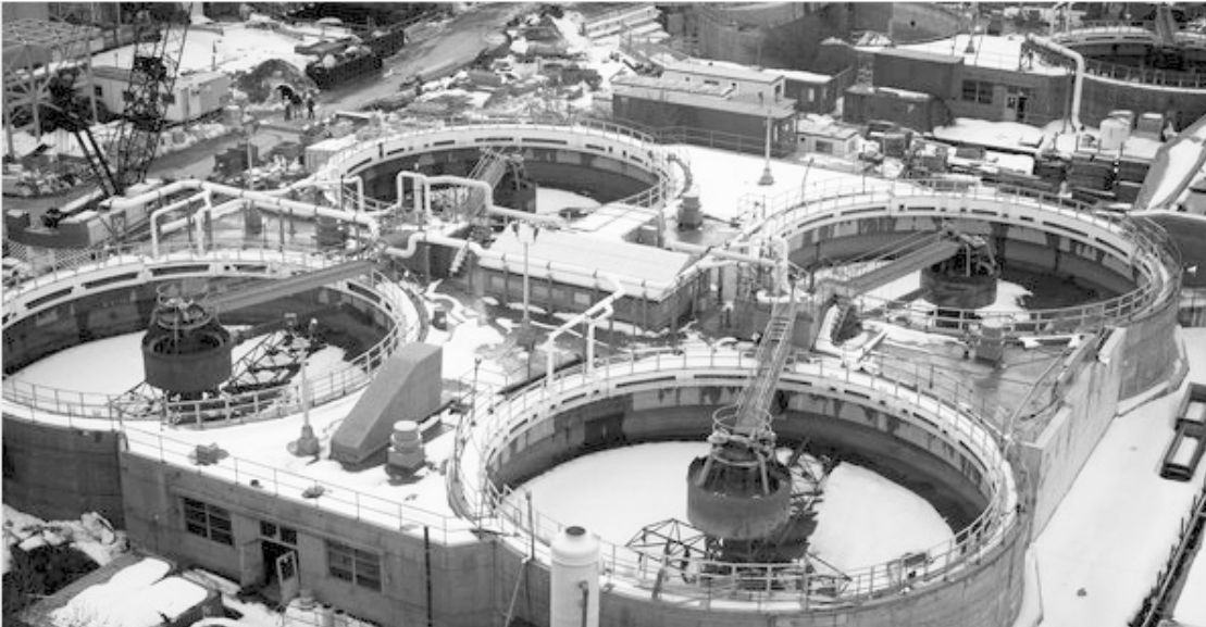
Fig. 2.0 New York City's Newton Creek Wastewater Treatment Facility in Greenpoint, Brooklyn photographed during construction.
