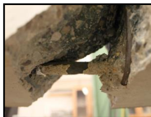
(e) Close up view of failure crack
