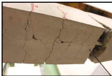
c) Splitting crack on left side
