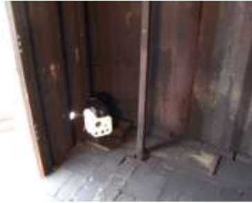
Figure 3-8 b. Volume Sensor Suite as Installed
