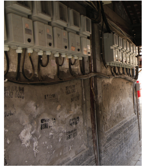
1.1.9 The number of meters installed indicates the number of families living within one courtyard house
