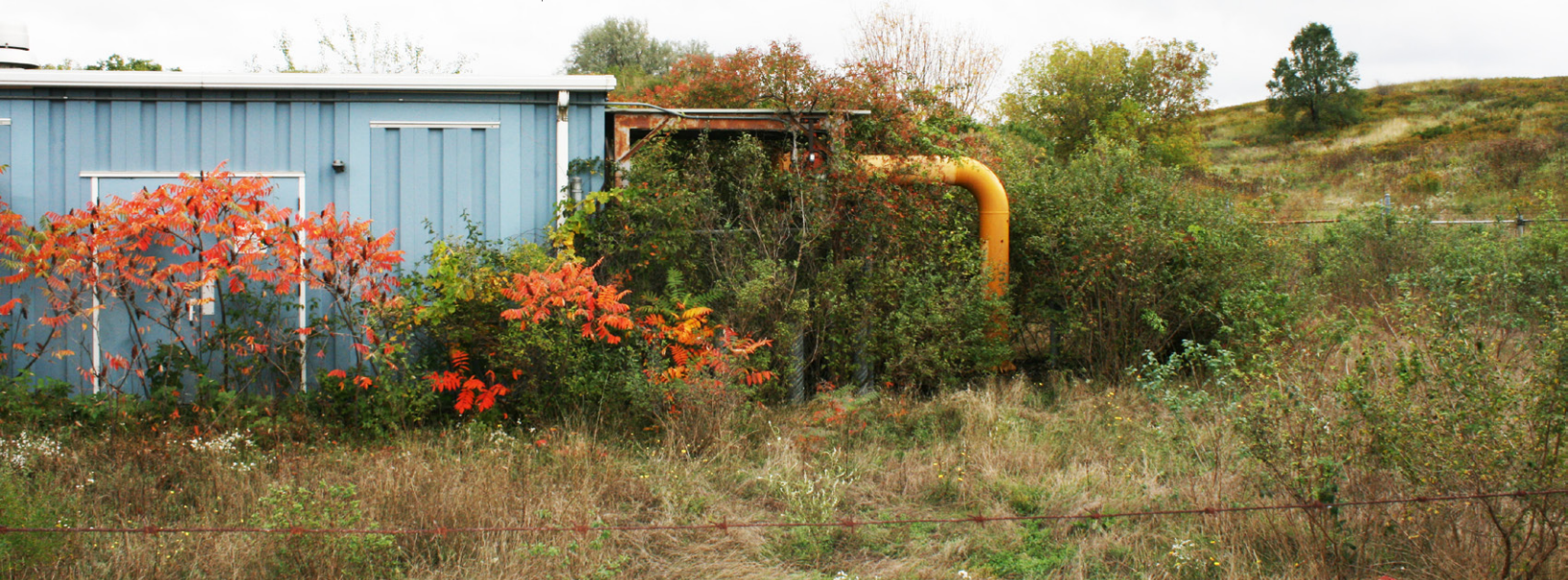
fig. 4.06 the overgrown landfill gas flaring facility at the Upper Ottawa Street Landfill
