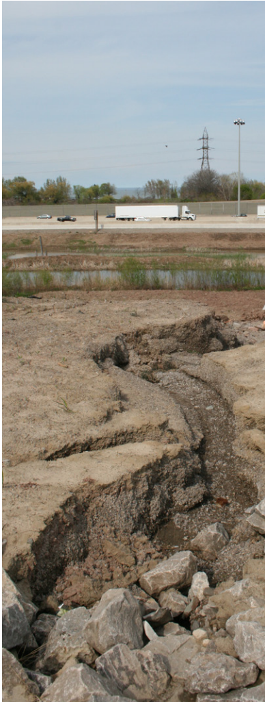
fig. 2.13 eroding cap at Brampton St. Landfill, Hamilton, Ontario
