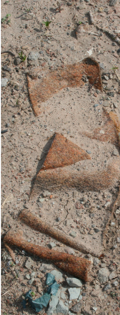
fig. 3.20 cap erosion unveils solid waste at Brampton Street Landfill
