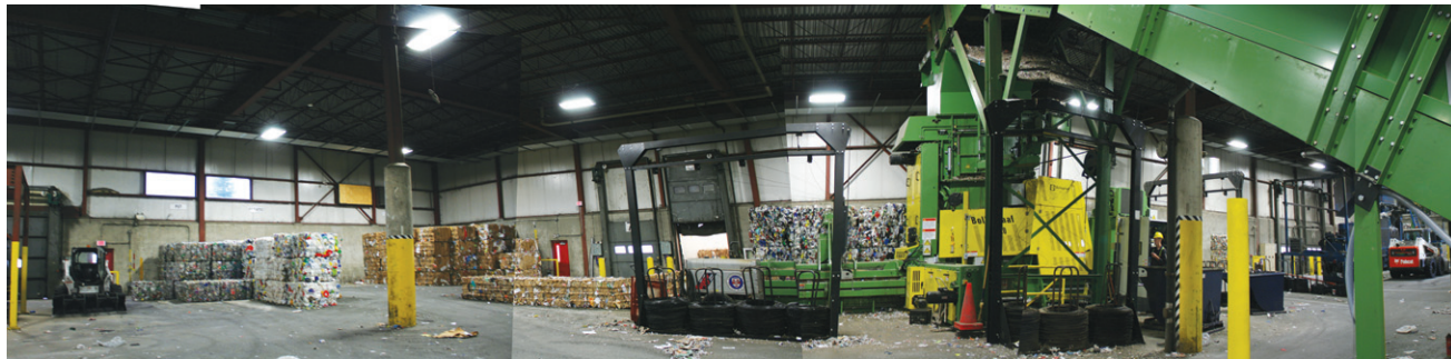
fig. 3.13 Compacting, baling, and storing hall within the Guelph Material Recovery Facility in Guelph, Ontario
