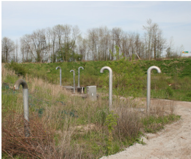
a 201 gooseneck vents in the Brampton St. Landfill
