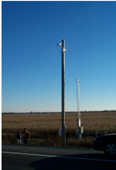
(a) Sensor Installation
