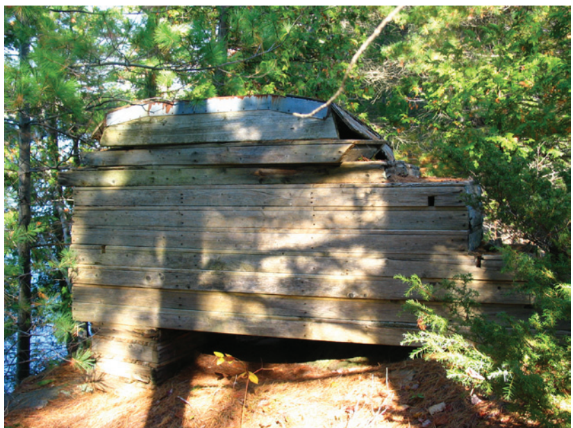
Fig.99: The old wood formwork for the concrete walls remain on the island.
