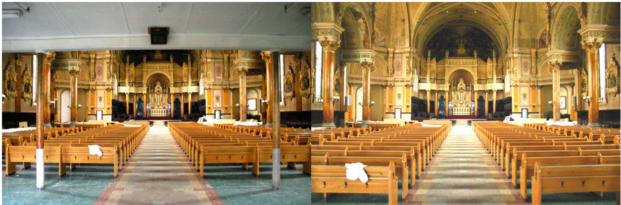
Fig.2.22. View towards the apse: obstructed by the tribune above (left) and unobstructed (right)
