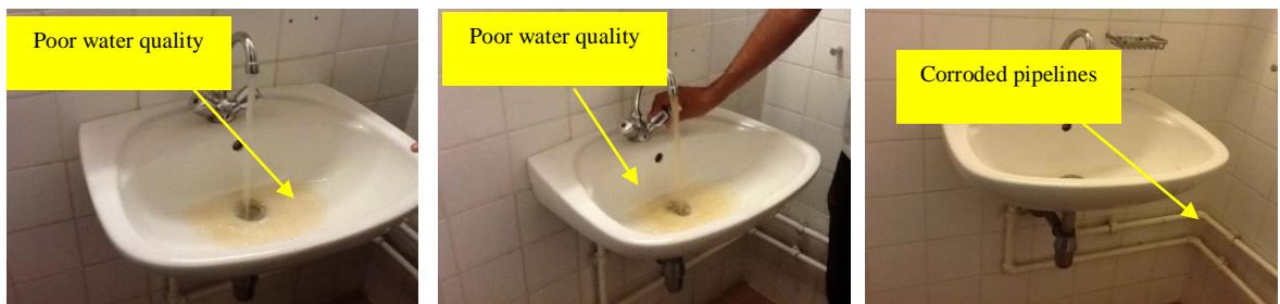
Figure 5.14: Poor water quality due to corroded pipelines
