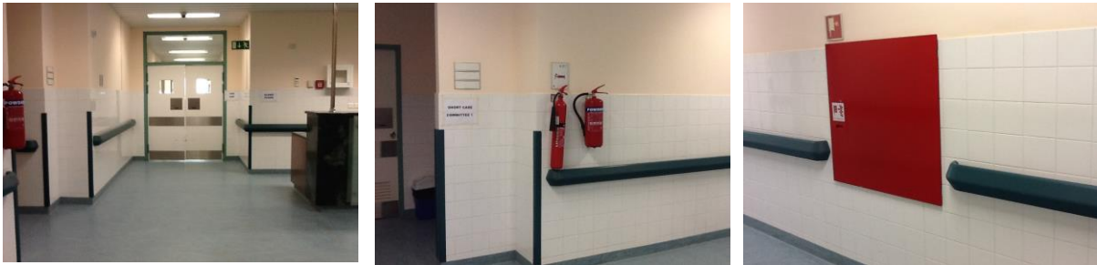
Figure 5.16: Fire alarm system
