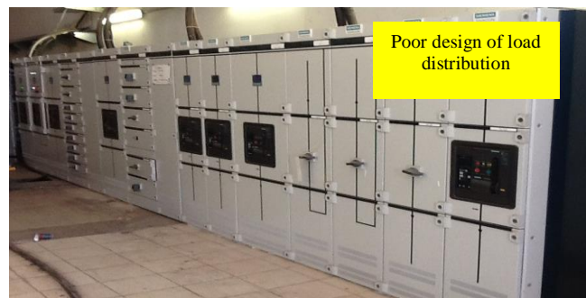
Figure 5.12: Problems with the low-voltage switchgear (electrical distribution)
