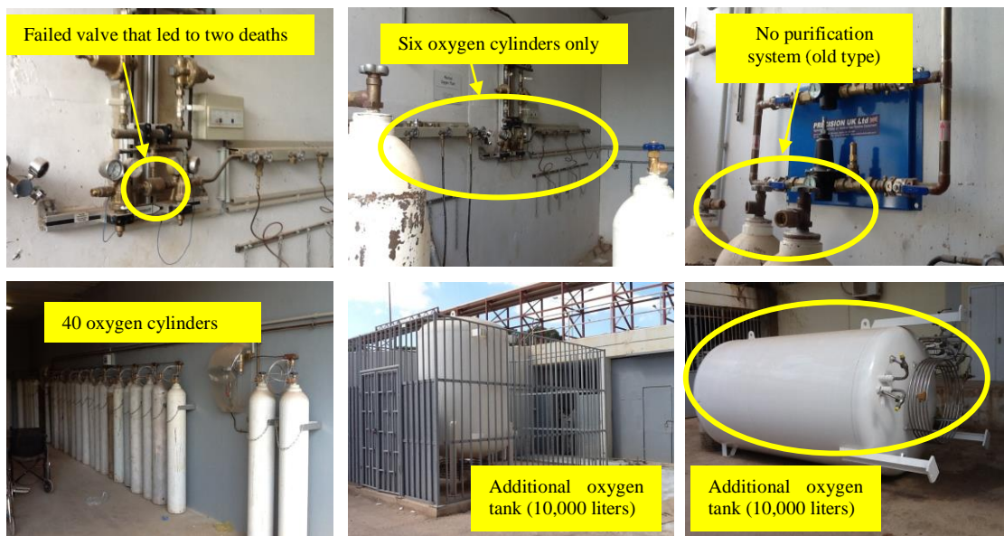
Figure 5.9: Problems with the medical gases system
