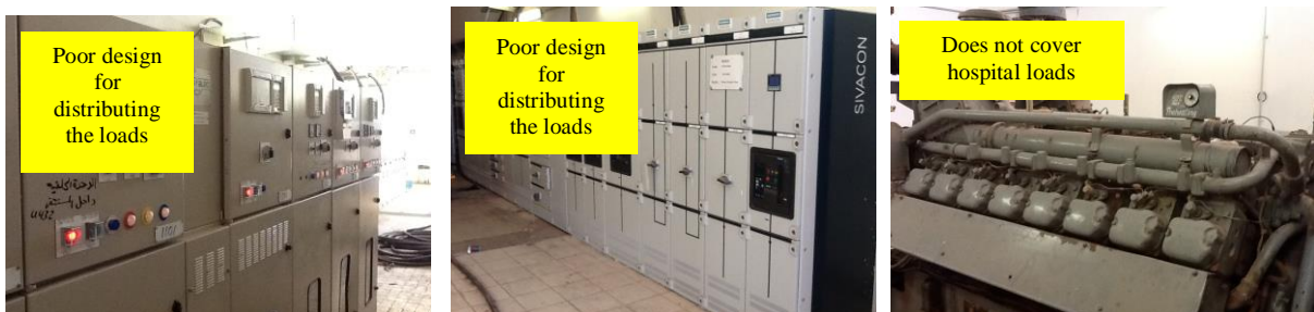
Figure 5.11: Problems with the high-voltage switchgear subsystems
