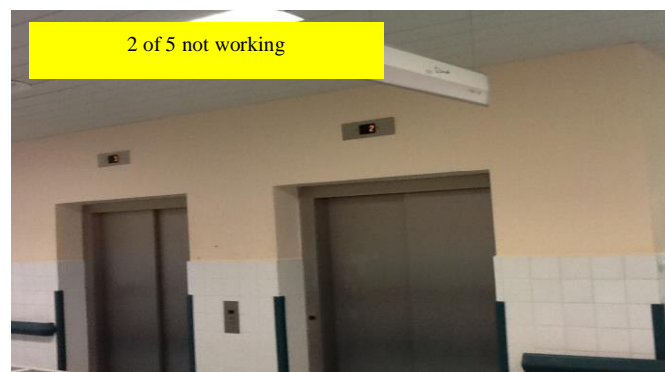
Figure 5.13: Elevator problems (2 of 5 not working)
