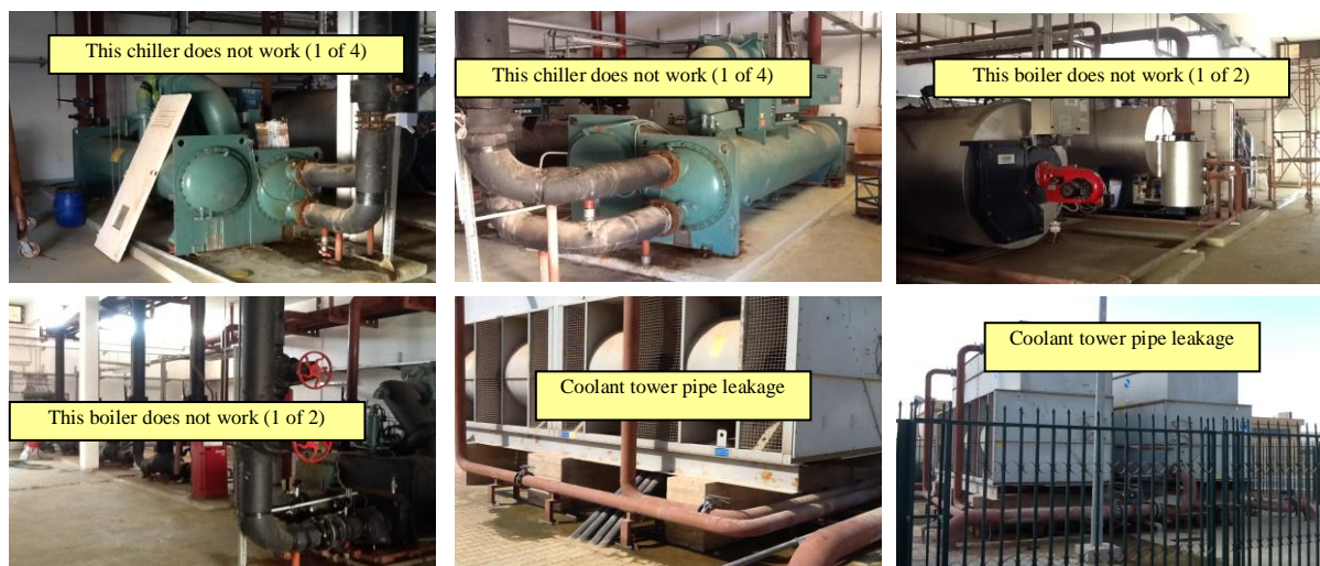
Figure 5.8: Problems identified in the boilers, chillers, and coolant towers
