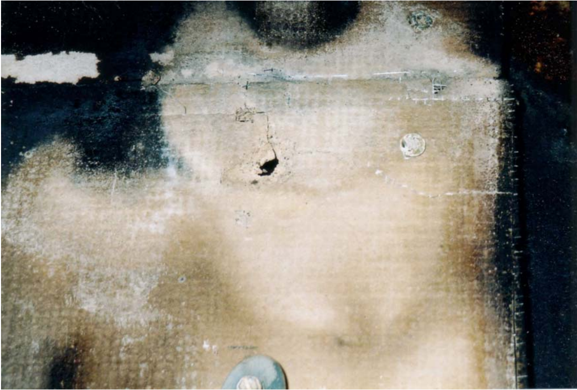
Figure 5: Evidence of Fire Penetration into an Exposed Sheet of Durock® Cement Board.
