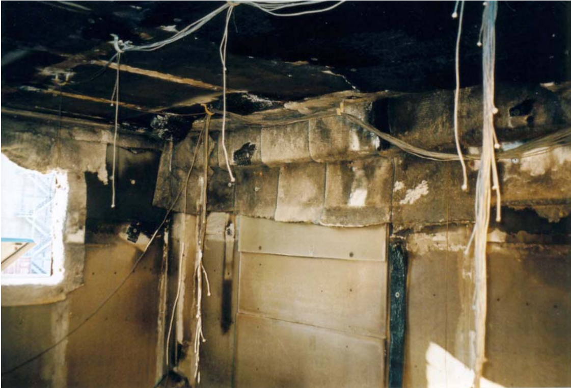
Figure 4: Room Condition after the 4th Burn, Nov. 25/04 with a view into the SW Corner.
