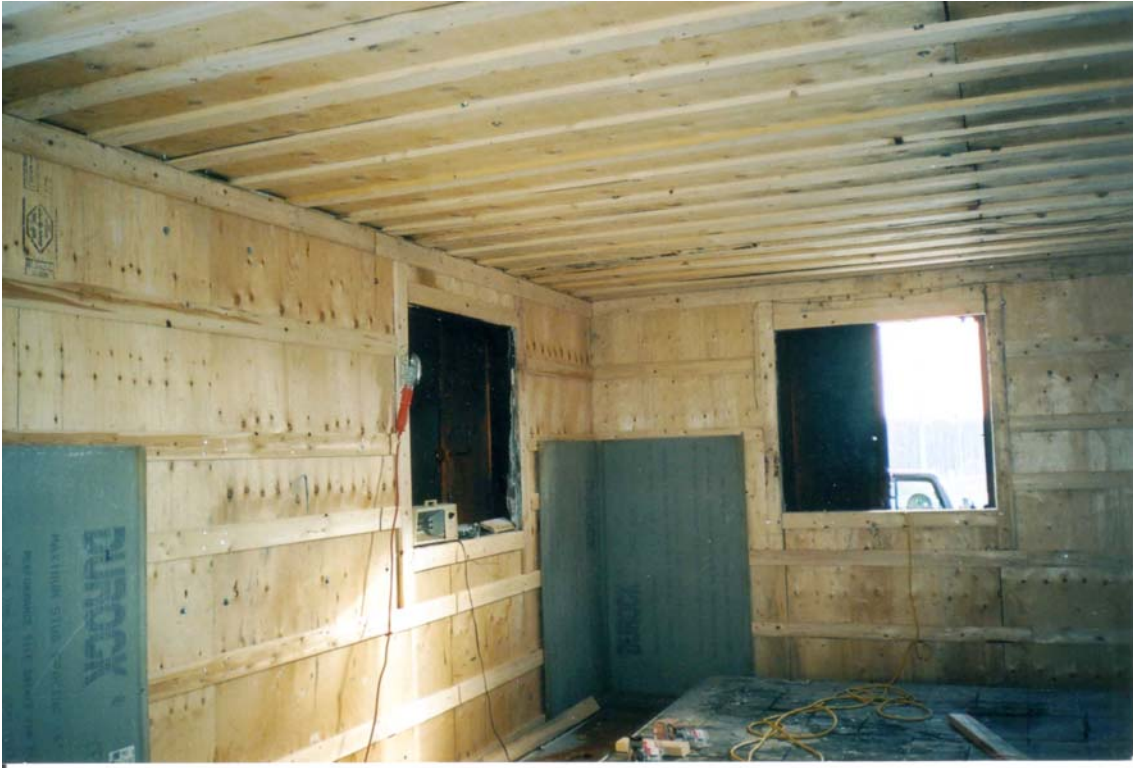
Figure 2: Burn Room Liner under Construction Showing Plywood, Strapping and Partial Installation of Durock Concrete Board. (South Wall in the Background)
