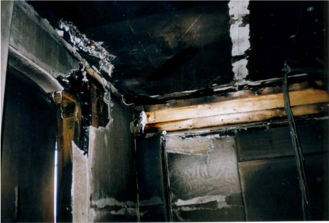
Figure 3: Room Damage After the 2nd Burn, June 20/04 Showing the Result of Fire Penetration Through the Wall at the Top Corner of the S Window and the Area of the Boxed in Sprinkler Pipe.
