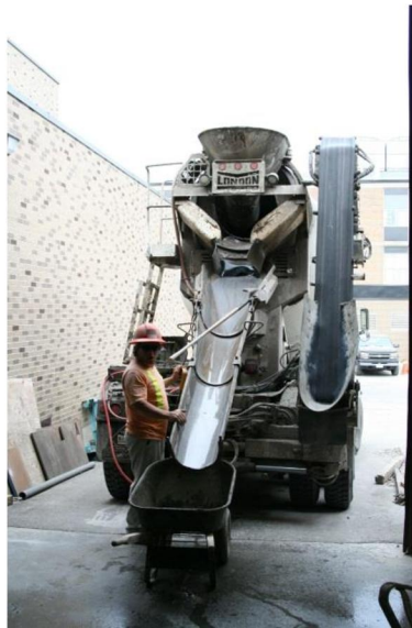
Figure 3-3: Mixer truck for concrete
