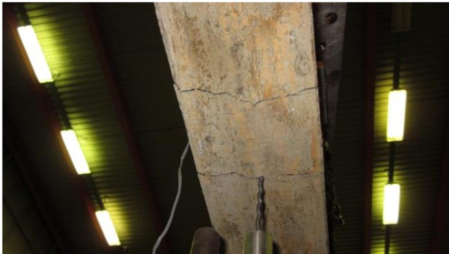
Figure 4-3: Average crack width for specimen 1
