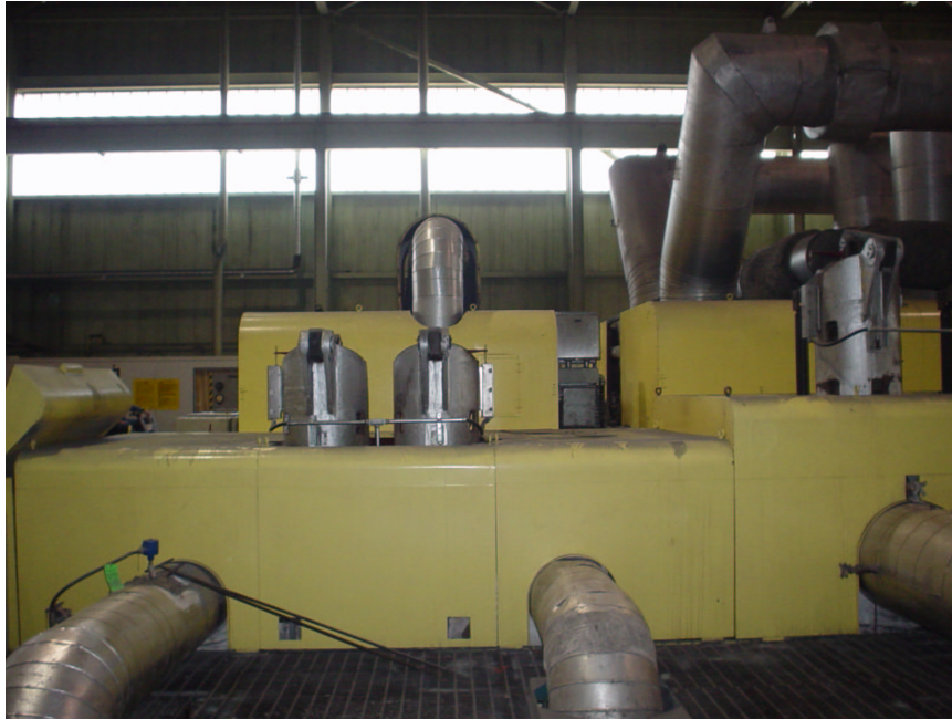
Figure 5.5: High-pressure section of Nanticoke turbine
