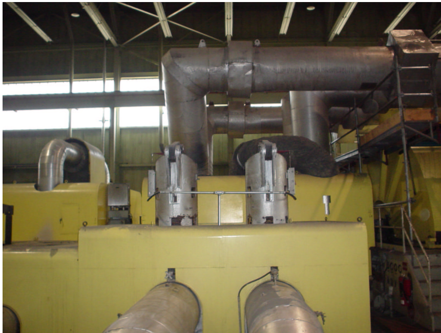
Figure 5.6: Intermediate-pressure section of Nanticoke turbine
