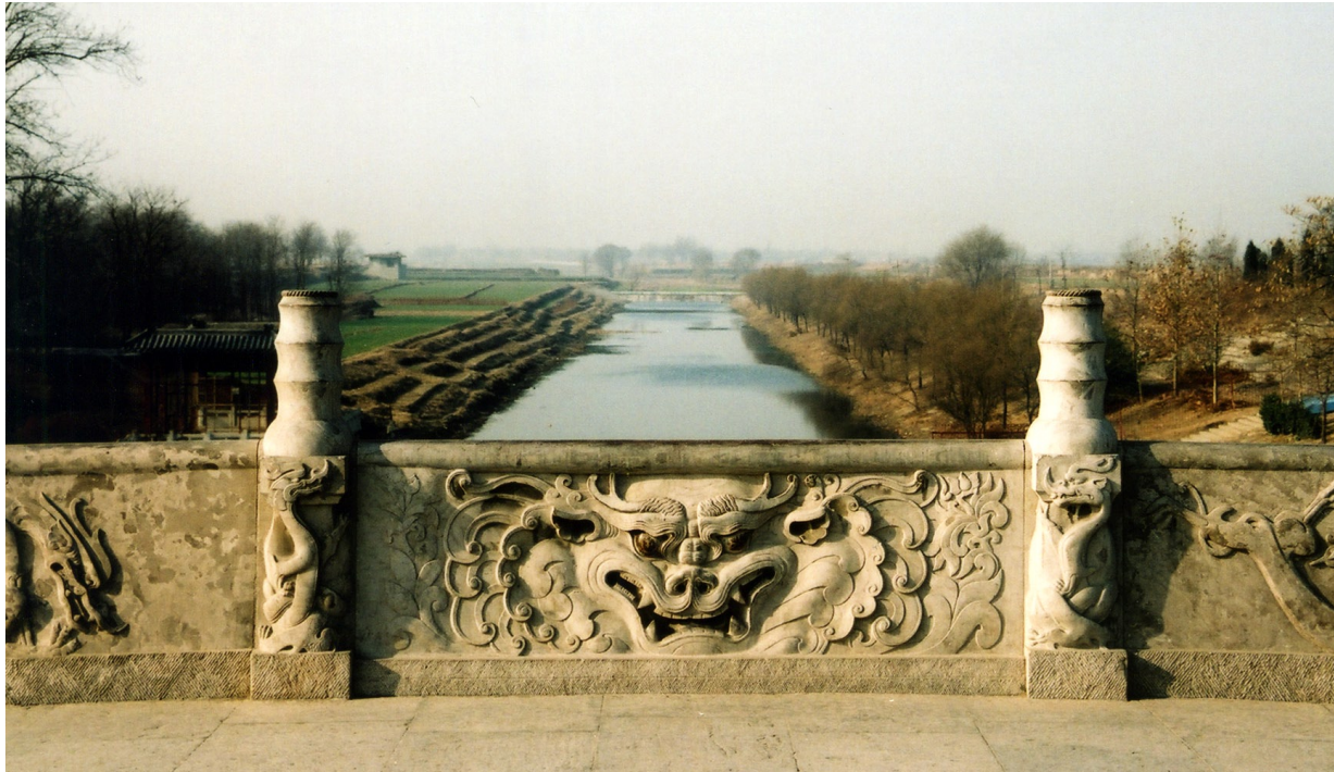
Fig. 11.2 Many scholars have condemned the restored bas-relief on the balustrade of the Anji Bridge as too clean and modern.
