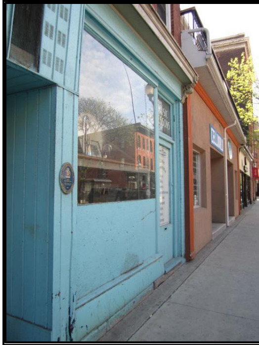
(Figure 17: View of designated heritage building with very poor building conditions in International Village, displaying Plaque)
